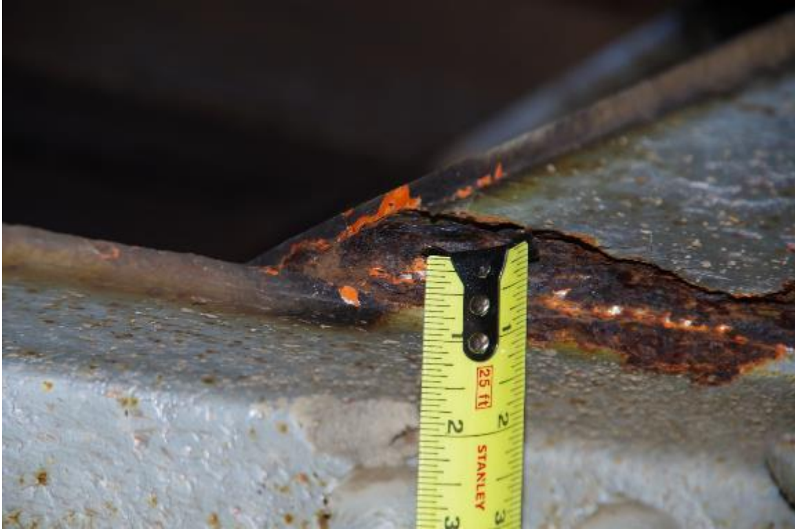
Photo 13: Closeup view corroded connection.
