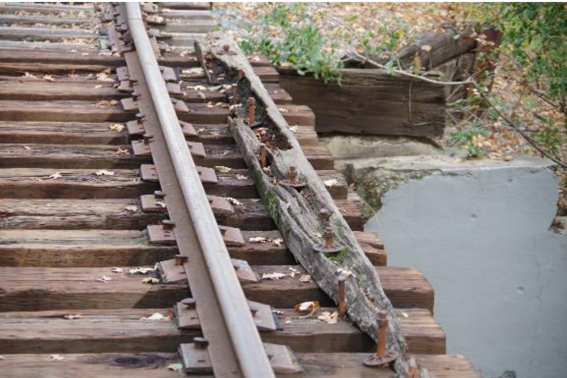
Photo 12: Right side of track. Tie keeper in critical condition.
