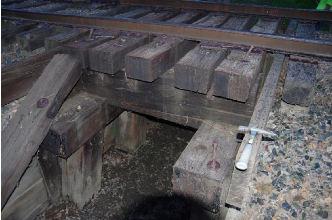
Photo 5: Closeup of railroad ties, timber girder, and bents. All are in fair condition.
