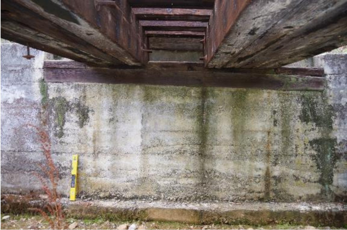
Photo 3: Abutment 1 typical section view. Seat width was measured to be 12 feet wide. Abutment 1 wall batter was determined to be 1 1/8"/ft
