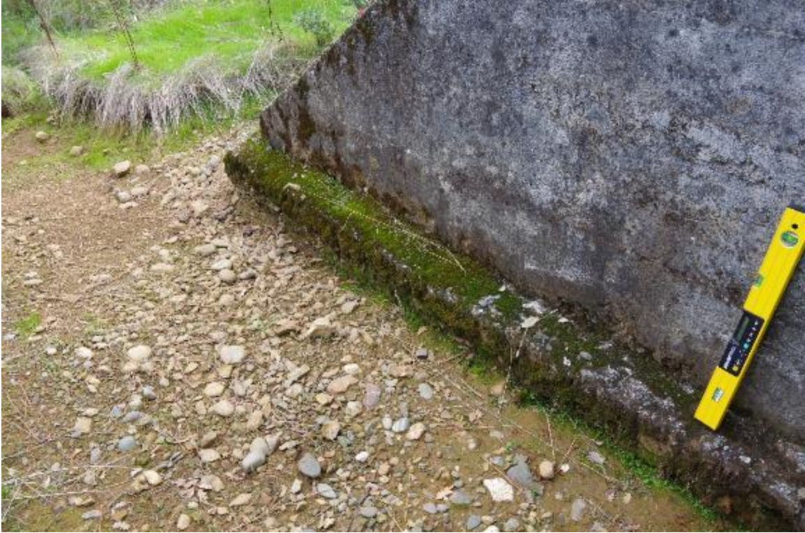
Photo 5: Exposed footing at Abutment 1. Footing sticks out approximately 6 inches.
