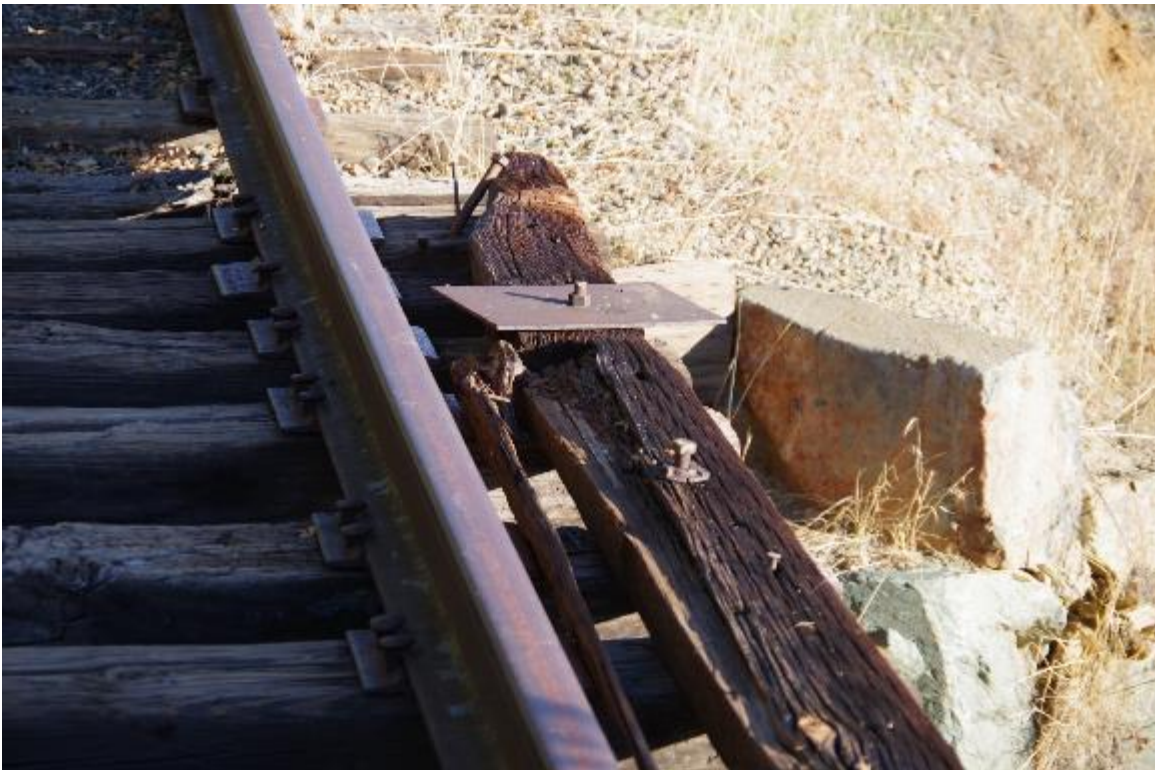
Photo 6: Tie keeper located on the right side of the track at abutment 2. Tie keeper is in critical condition due to age and timber falling apart.
