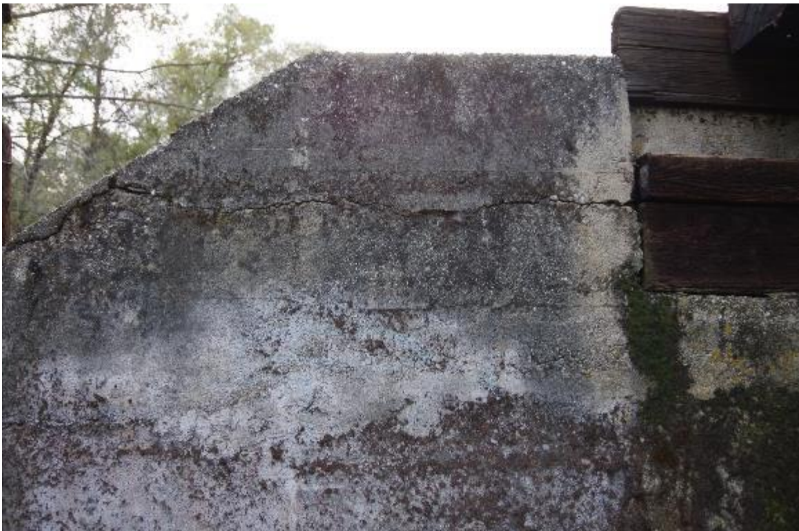
Photo 6: Closeup of left side of Abutment 1. Crack observed slightly above abutment seat.
