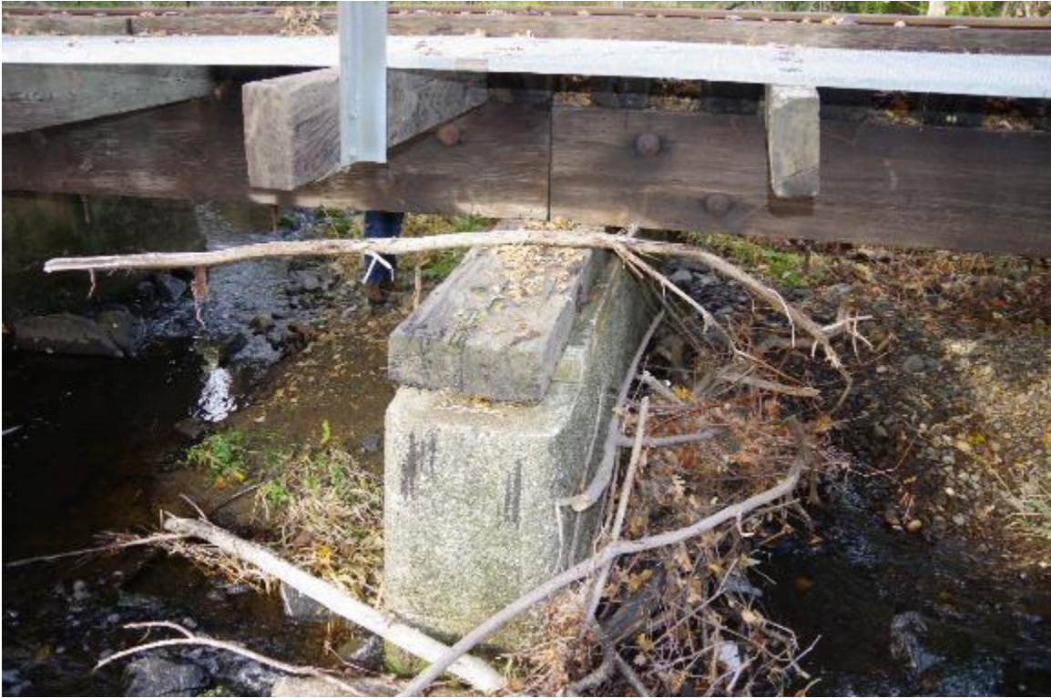
Photo 7: Closeup view of Pier 2. Semi continuous beams meet at this pier. Beams are sitting on sill beams.
