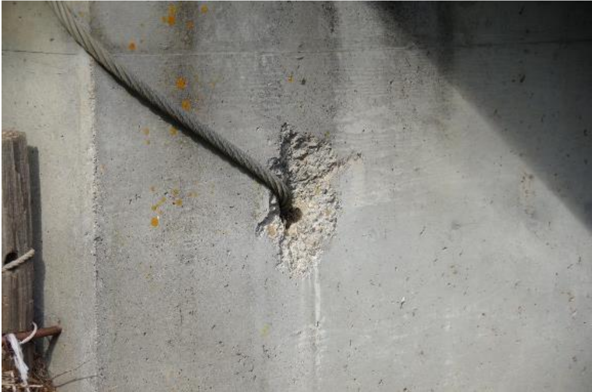
Photo 7: Typical seismic restrainer to Pier connection. Spalling at connection observed at most locations.
