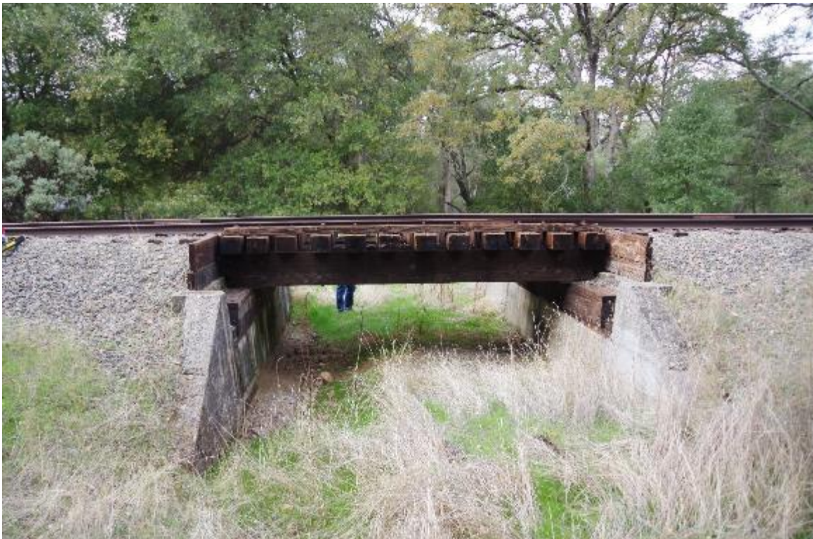
Photo 2: Bridge elevation view, right side of bridge. The single span of bridge is 15 feet. Slight vegetation through channel on both ends.
