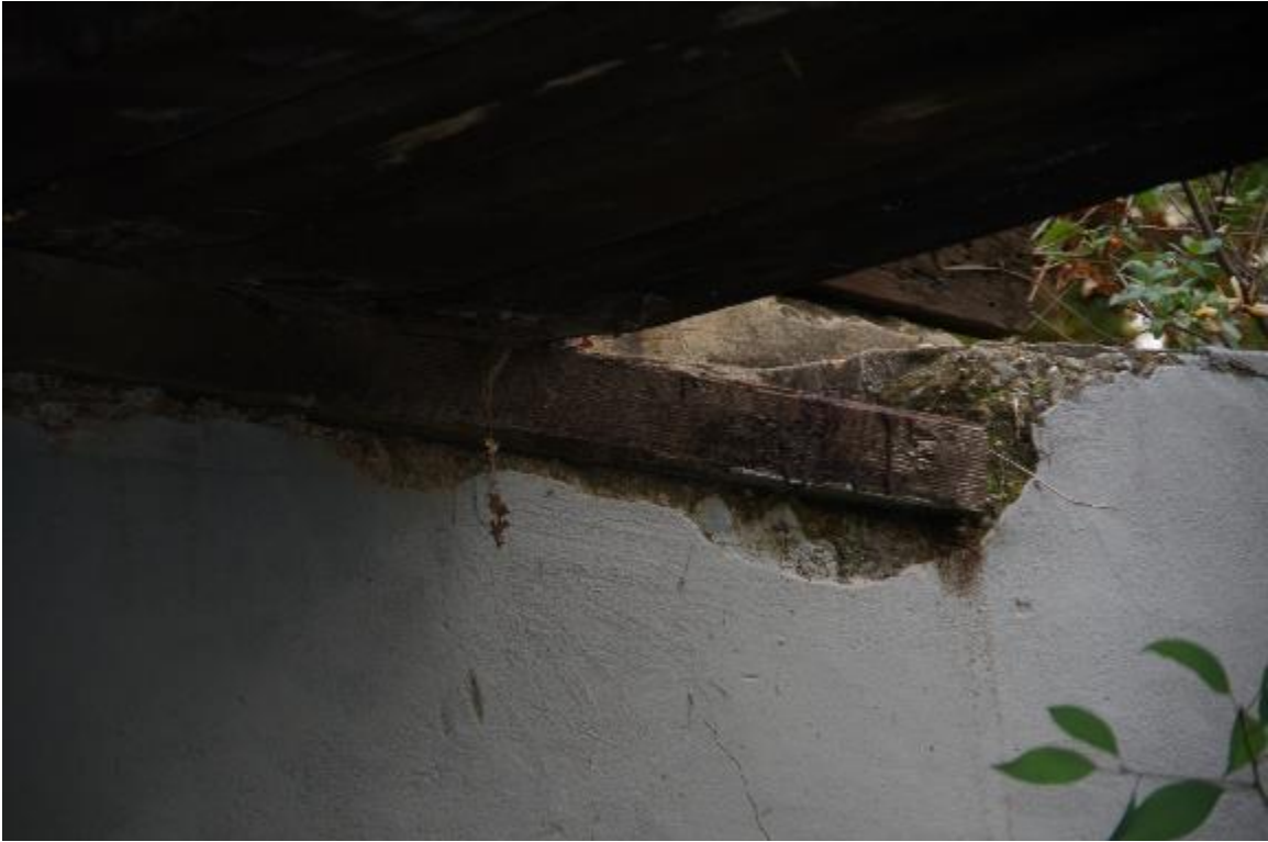
Photo 9: Closeup of concrete spalling at right side of Abutment 2.
