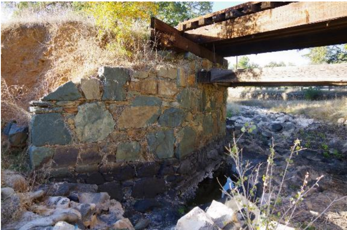
Photo 8: Embankment erosion on right hand side of Abutment 1.
