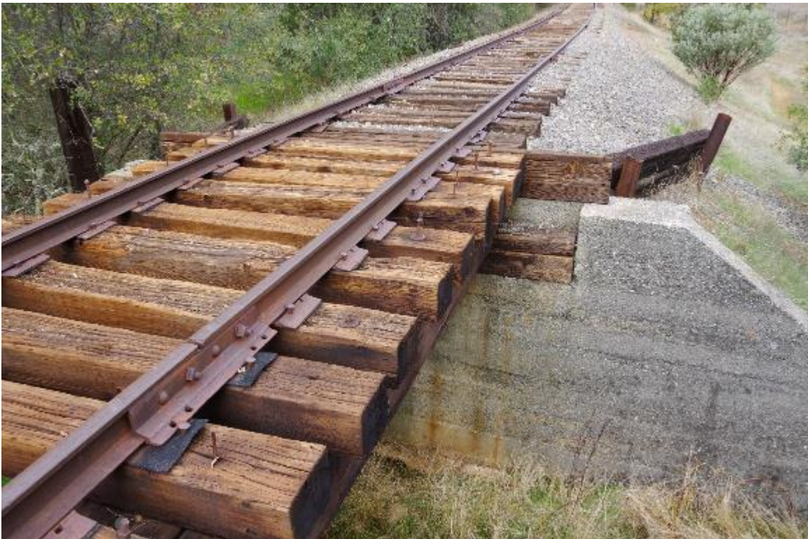
Photo 4: Closeup view of top of bridge. Railroad ties are in good condition. No tie keepers observed. Steel track is in fair condition.
