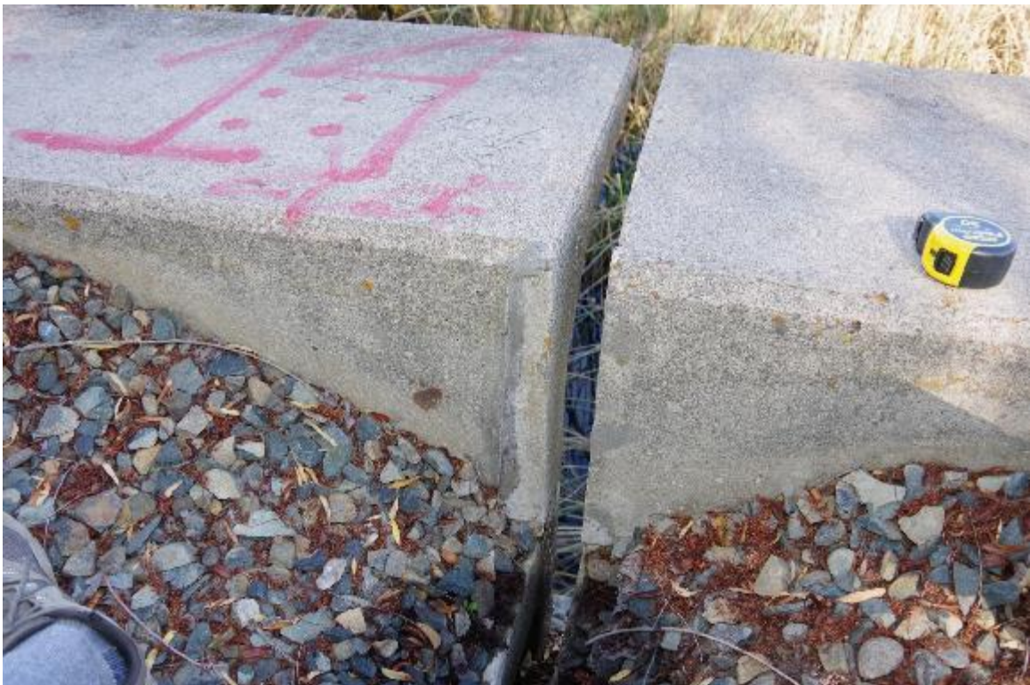
Photo 10: Typical joint opening between box girder spans. Ballast was found to be inside of these joints. Picture shown is the end of span 2. Joints are missing ballast cover.
