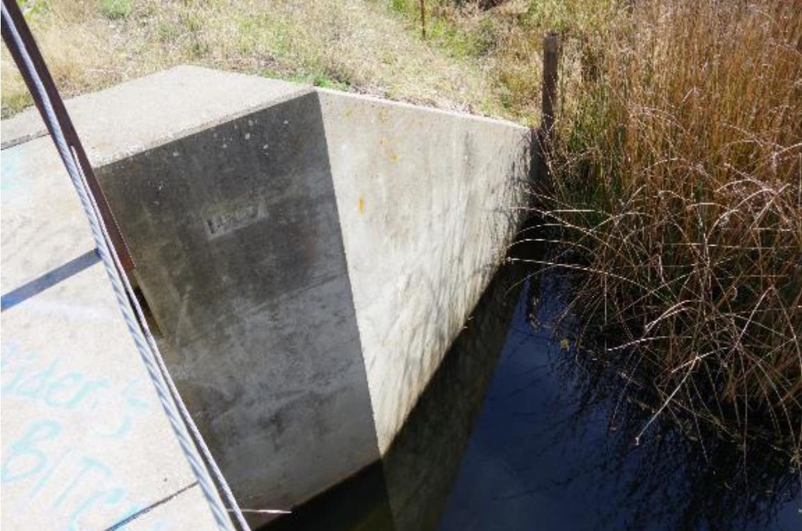
Photo 9: Right corner of Abutment 5. A date of 1967 is shown in the picture indicating year bridge was built.
