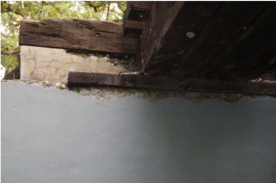
Photo 8: Closeup of concrete spalling at left side of Abutment 2.
