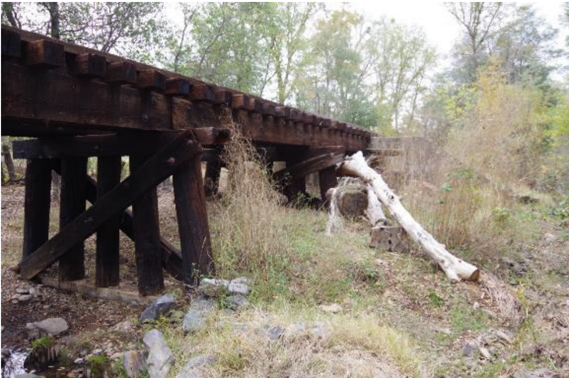
Photo 6: Bridge elevation view on right hand side. Pier 3 is shown. Pier 3 is in fair condition. Timber beams are semi continuous.
