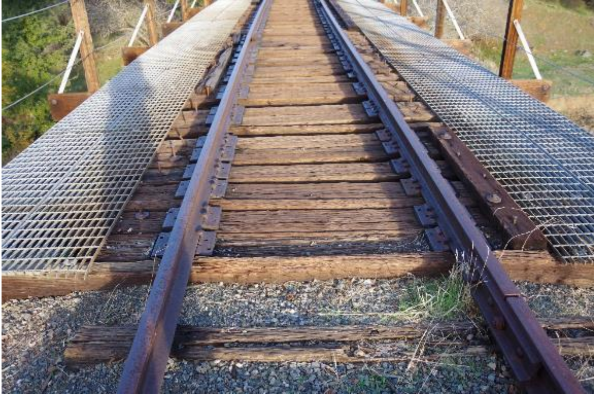
Photo 5: Closeup view of railroad ties, walkway supports, steel track. All are in good/fair condition.
