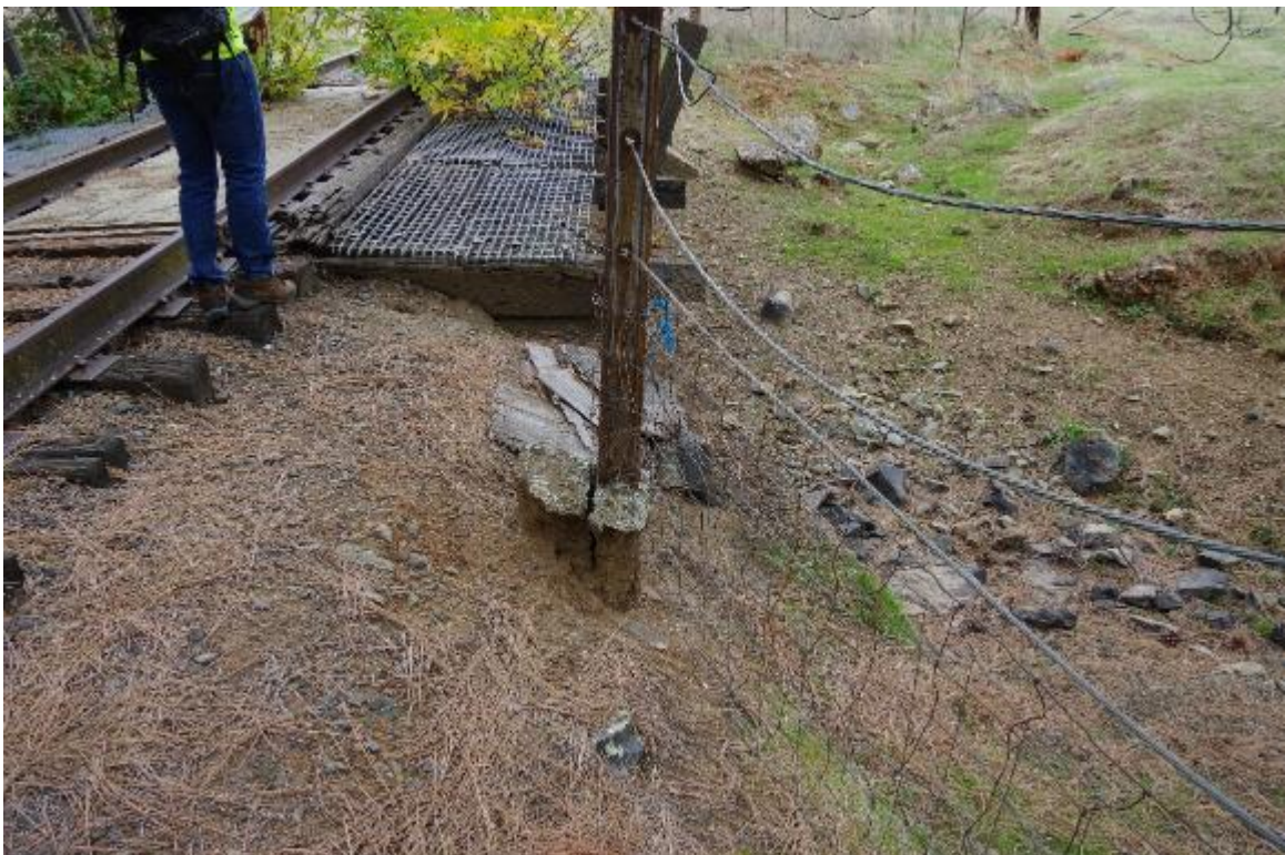
Photo 6: Closeup of damage post near Abutment 1. All other posts are in poor/critical condition.
