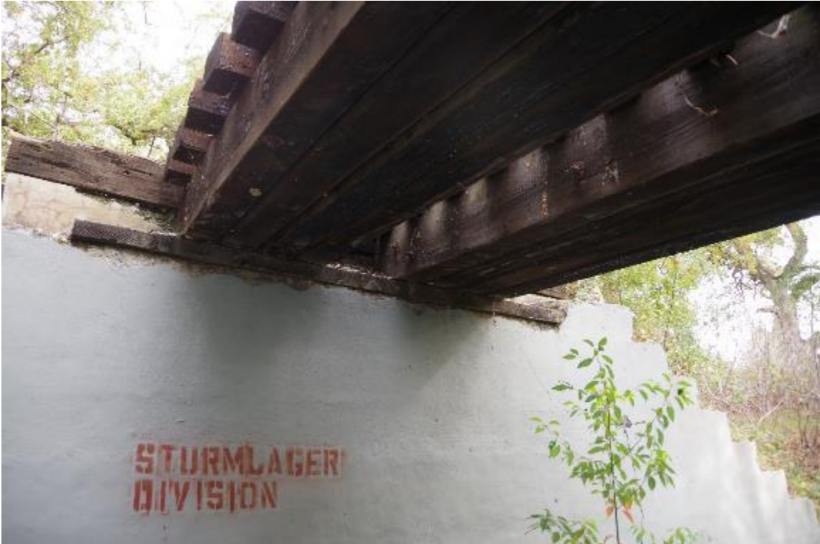
Photo 7: View of Abutment 2. Beams sit on 4"x 12" sill beam. A small amount of spalling shown at Abutment seat. Spalling also seen at headwall.
