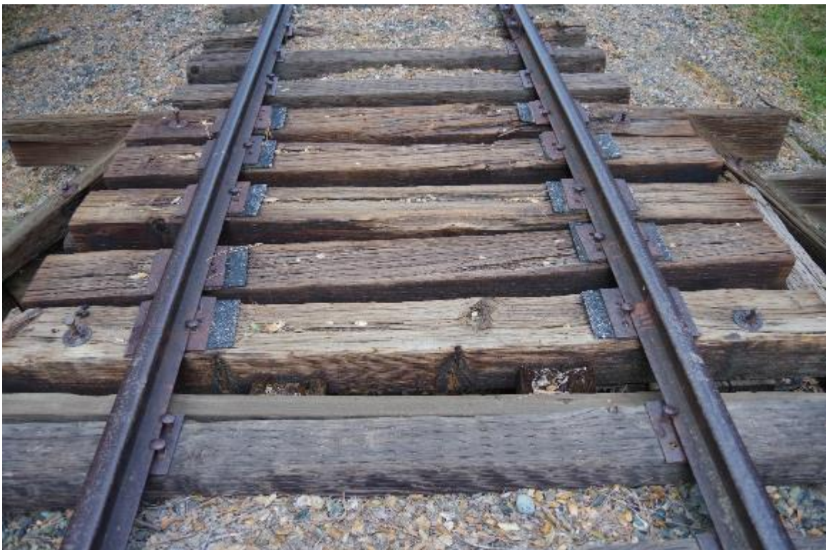
Photo 2: Close up view of track. Ties are in fair condition. Some minor damages observed due to age of ties. Steel track is also in fair condition.
