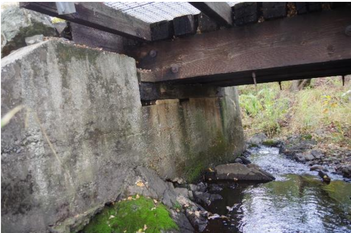
Photo 4: Abutment 1 shown. Large rock seen at the bottom of the left hand side. Abutment is on a superelevation. Walkway supports, Ties, and beams are shown.
