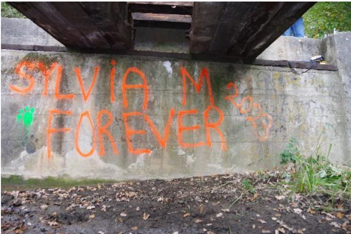
Photo 6: Abutment 2 section. Wall is in fair condition. Timber girders are also in fair condition.
