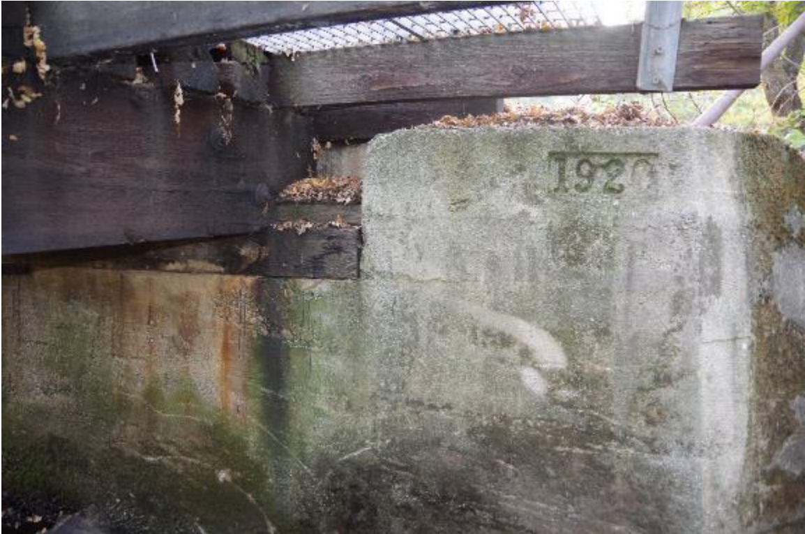
Photo 5: Right side of Abutment 1. A date of 1920 is shown indicating when the bridge was built.
