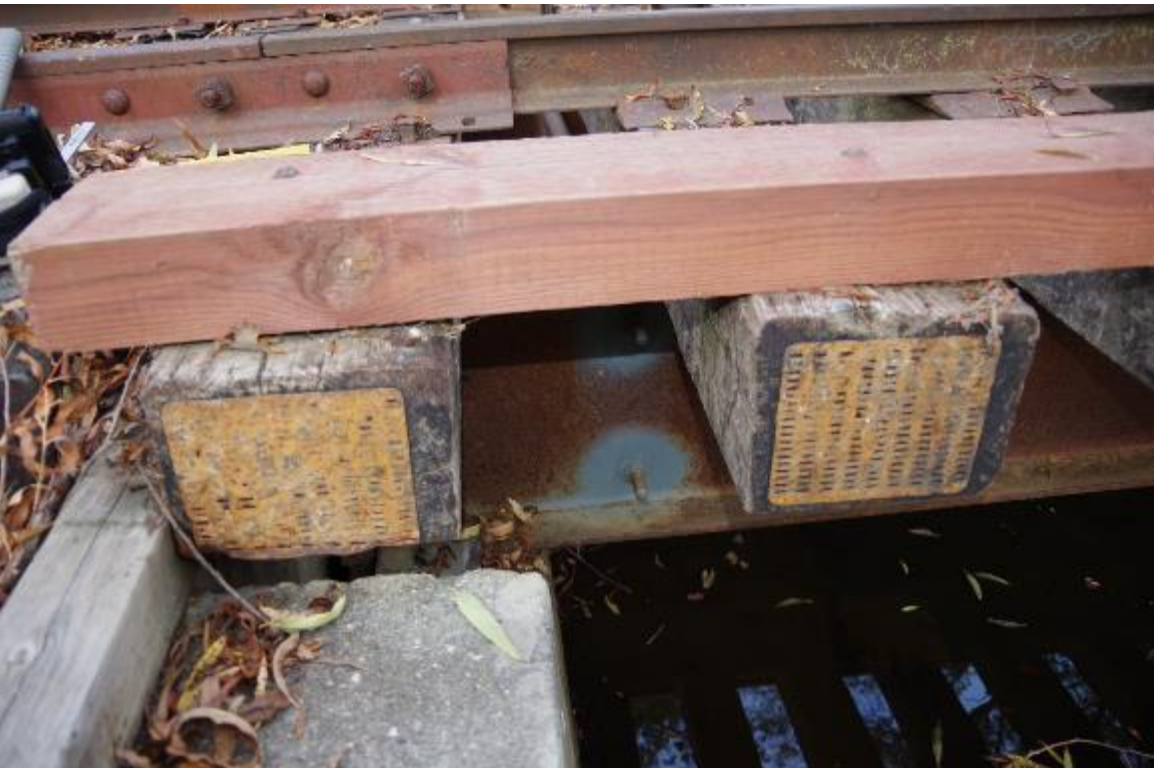
Photo 4: Close up view of steel girder, rail road ties, tie keeper, and rail track. Rail road ties and steel girder (ASTM A992) are in good condition. Tie keeper is relatively new.
