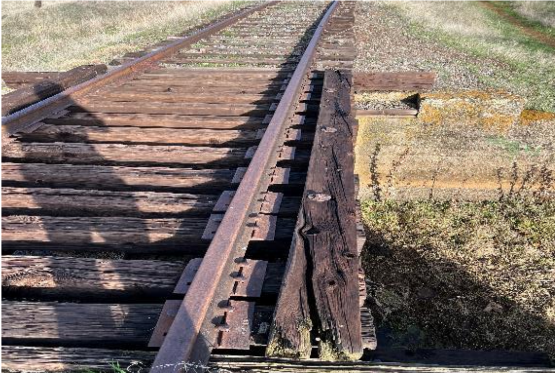
Photo 3: View of top of bridge showing condition of railroad ties, steel track, and tie keeper
