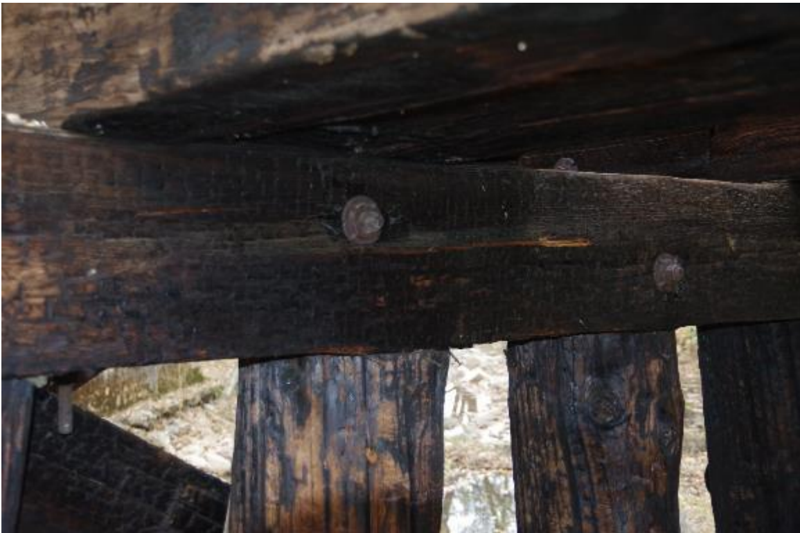
Photo 4: Close up of bent cap at Pier 2. Bent cap is clearly charred from a past fire. Columns also appear to be affected.
