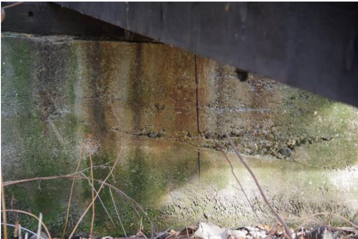
Photo 12: Closeup of Pier 3. Concrete spalling observed on the battered wall.
