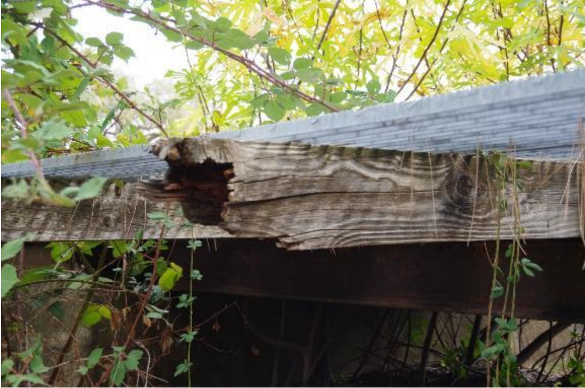
Photo 5: Close up of a damaged walkway support on left hand side of bridge, span 1.
