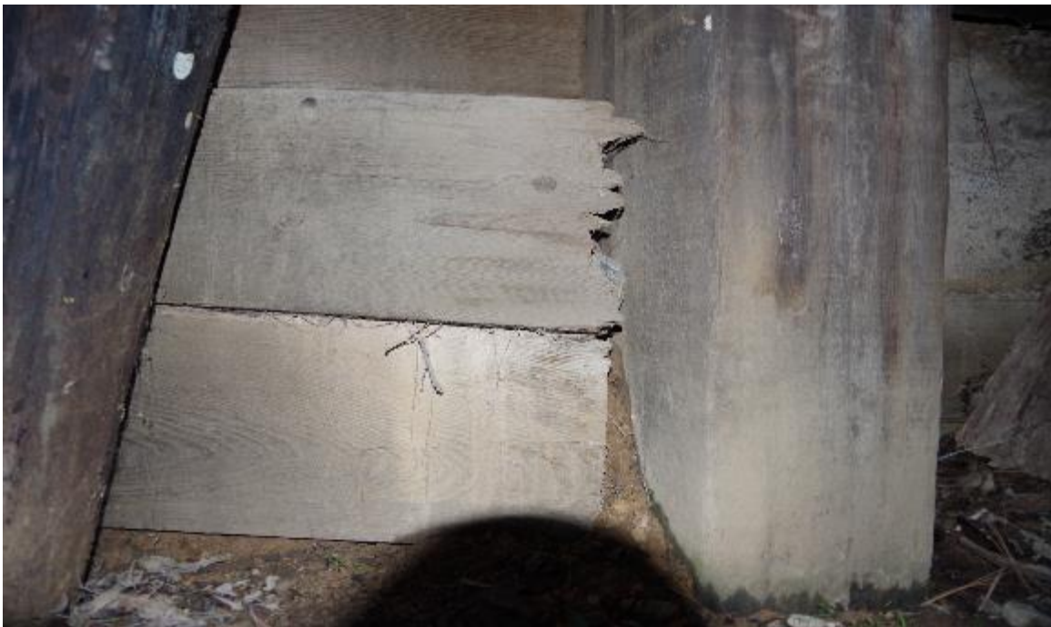
Photo 4: Close up view of timber lagging at Abutment 1. Lagging is in poor condition due to damage and movement. A small amount of embankment fill can be seen pushing through lagging.
