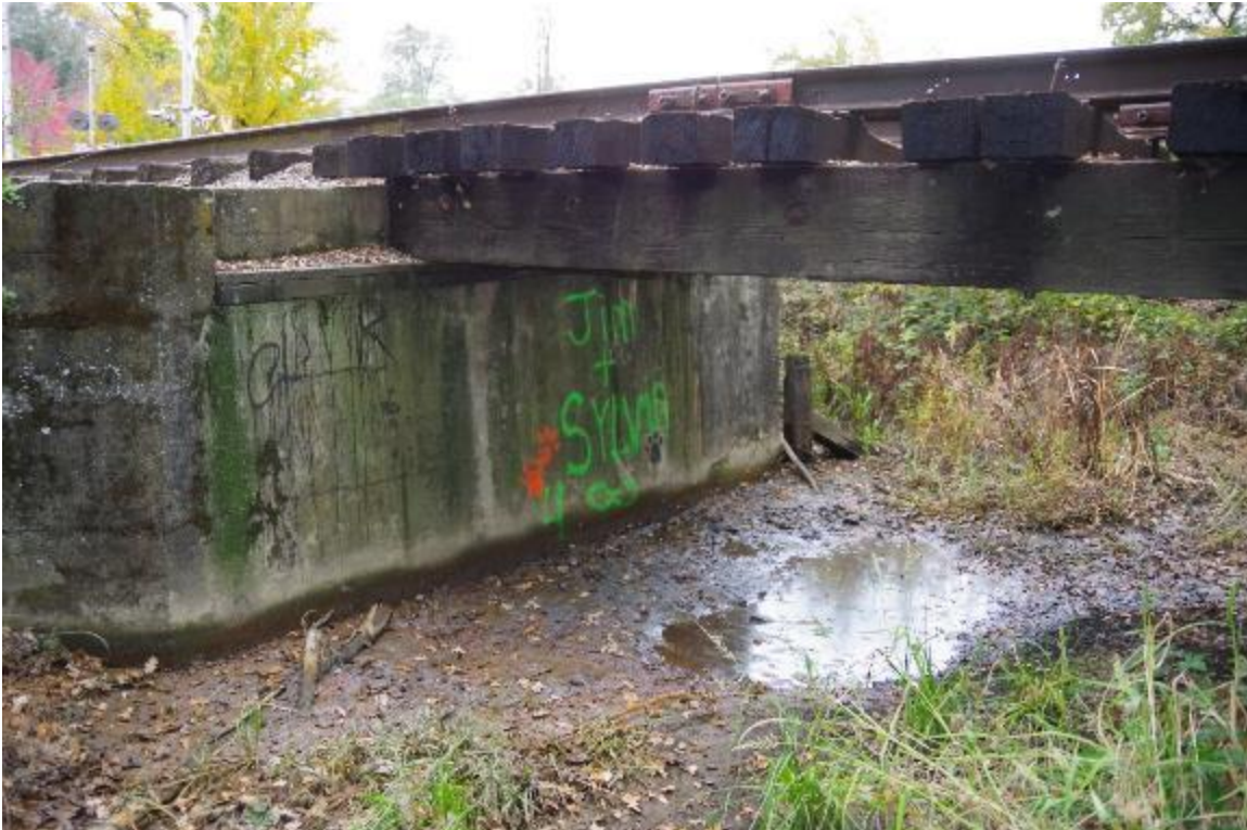
Photo 5: Abutment 1 view. Height of abutment measured as 4'-6". Wall has a batter of 1 1/8"/ft. (Abutment 2 similar). Abutment 1 has a 3° super elevation and Abutment 2 has a 4° super elevation.
