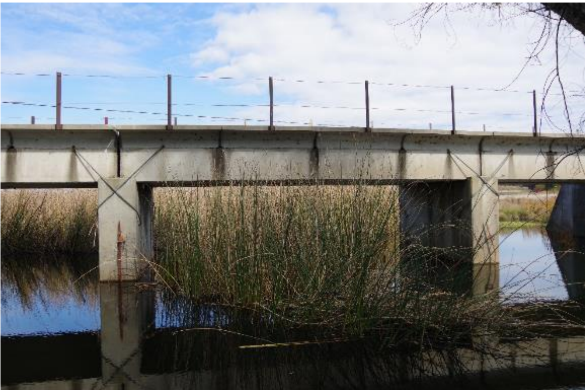
Photo 2: Bridge elevation view from east side of track, Pier 3 & 4 shown. Typical span is 30 feet.
