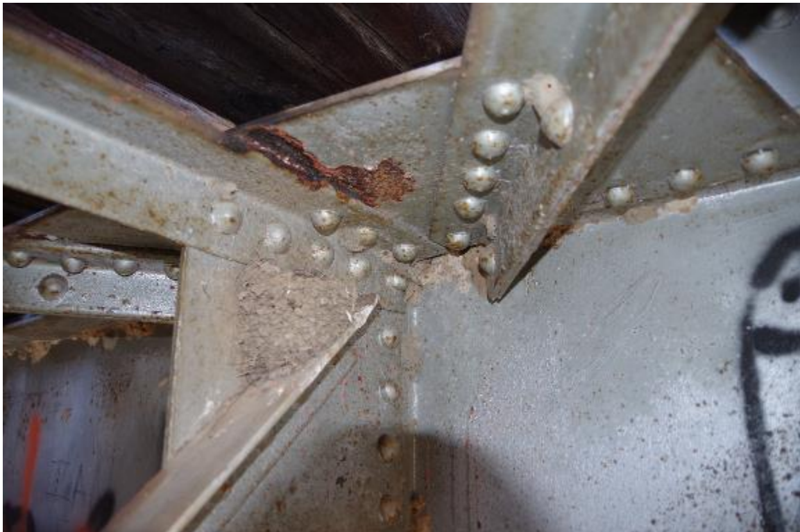
Photo 12: Gusset Plate Connection Pack Rust Corrosion
