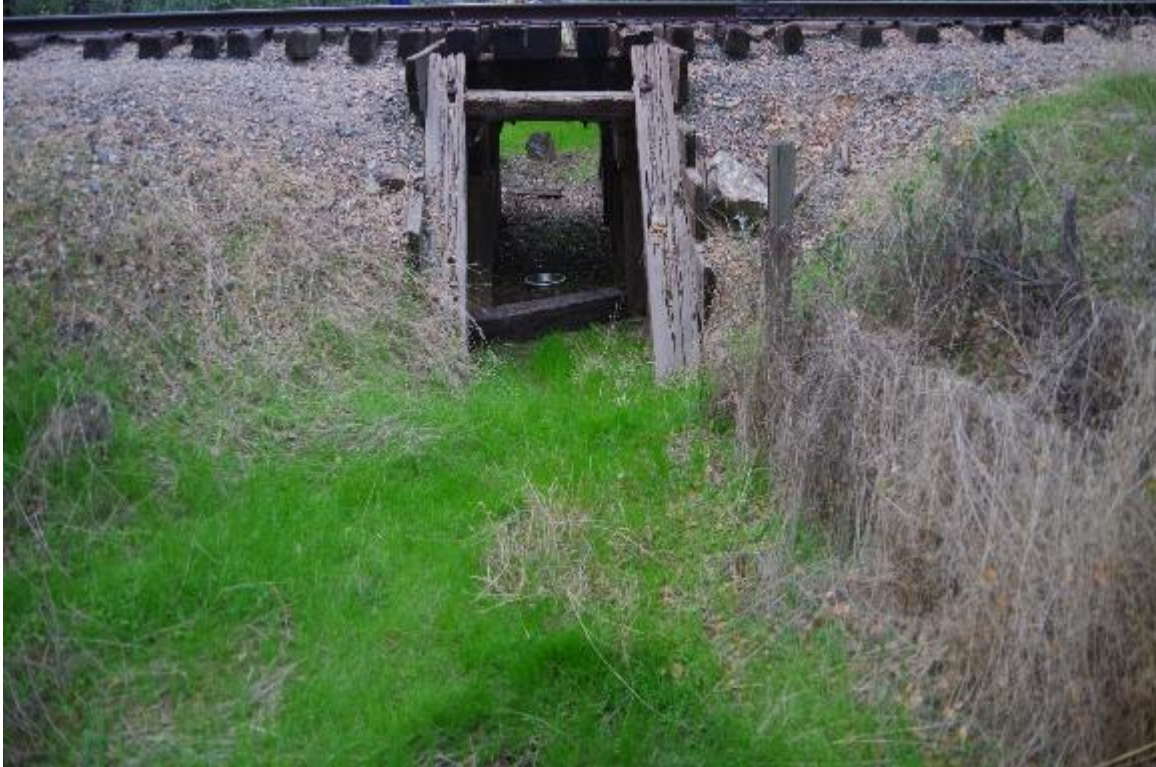
Photo 3: Bridge elevation view, photo shown to the right of track. Bridge length is 4'-6".
