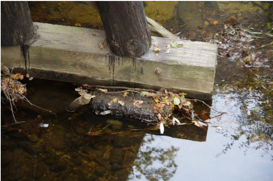
Photo 4: Close up view of Timber beam sitting on a concrete footing at Pier 2.
