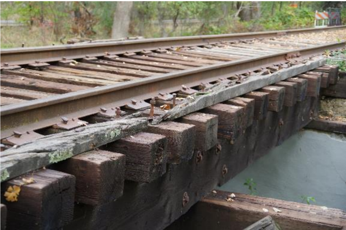
Photo 4: Close up of bridge on the right side. Railroad ties are in poor condition and timber airder are in aood condition. Tie keepers are in critical condition. Bolts are exposed.
