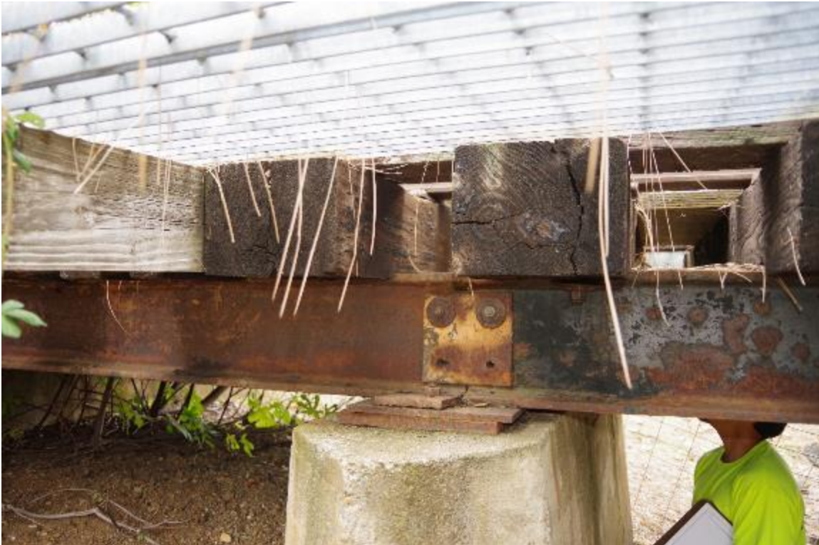
Photo 3: Closeup view of steel girder connection at Pier 2. Steel in moderate/poor condition due to rust. Paint on the beams is in fair – failed condition throughout. Two bolts missing at plate connection. 2 span bridge.
