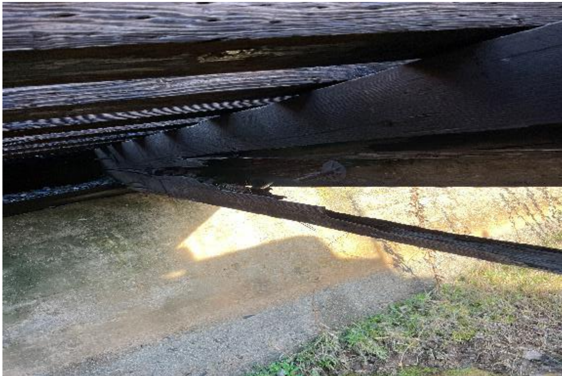
Photo 6: Closeup view of damaged girder.
