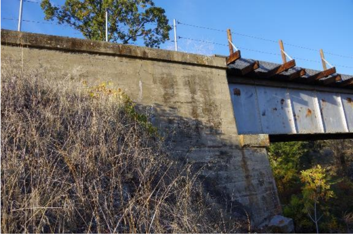
Photo 3: Closeup view of Abutment 1, right side of bridge. Large crack can be seen at the edge of the concrete headwall.
