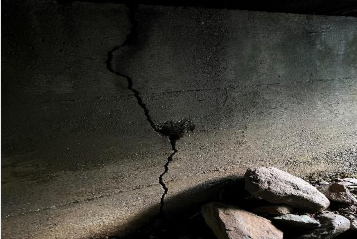
Photo 9: Abutment 1 diagonal crack
