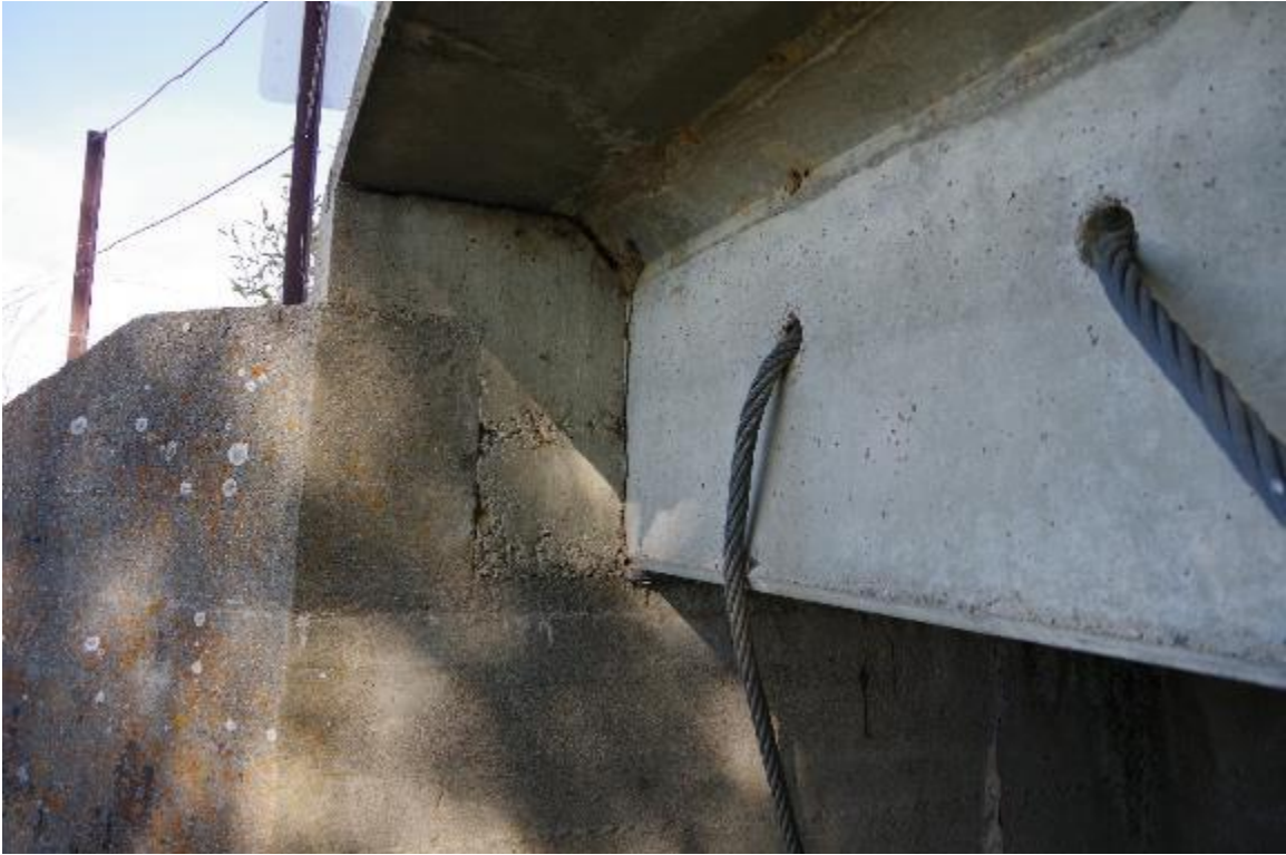
Photo 5: Closeup view of Abutment 1 and concrete slab connection. Shown are seismic restrainers.
