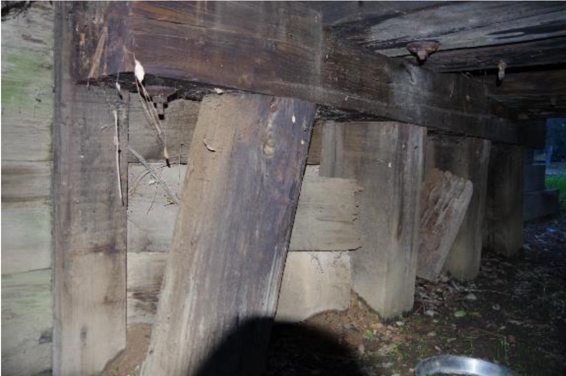
Photo 3: Closeup of Bent 1 near Abutment 1. One circular timber column, rest are square columns.
