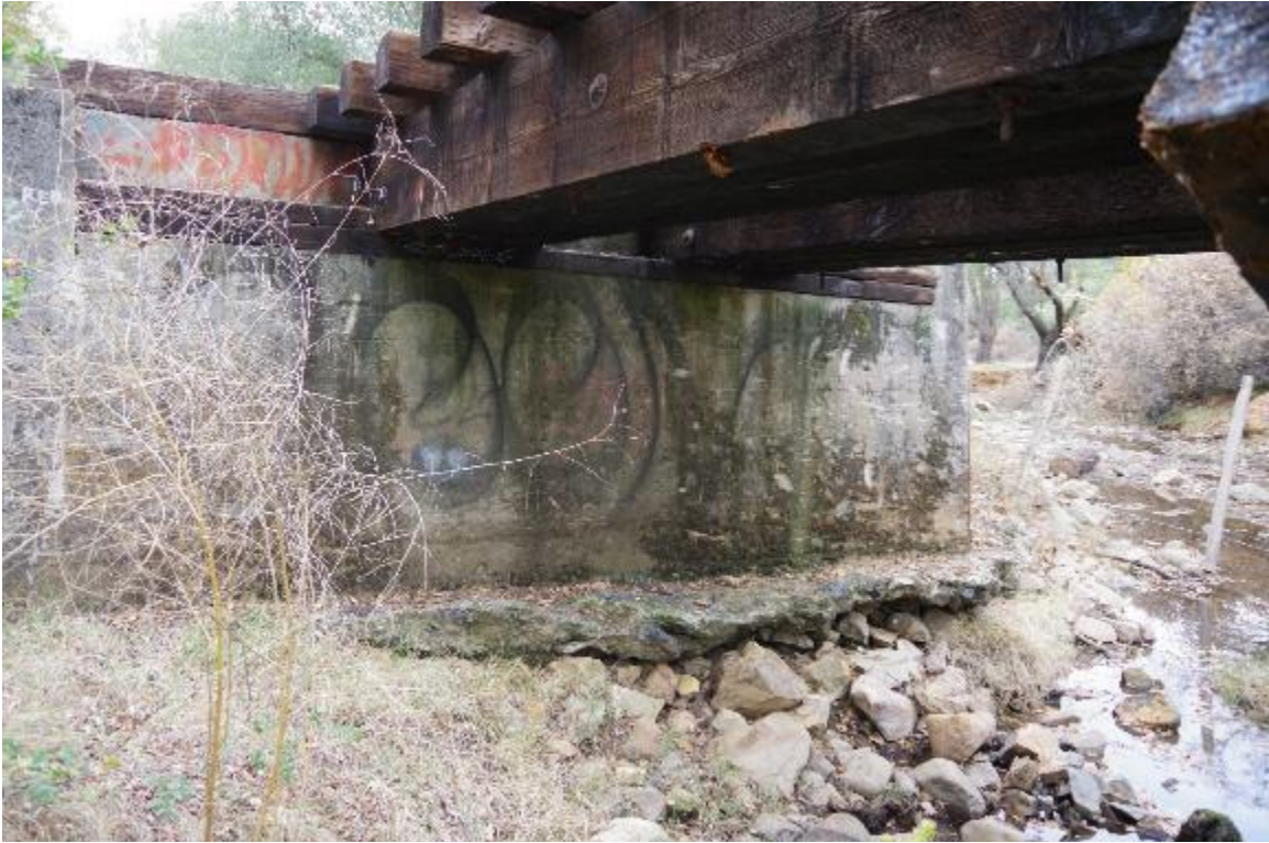
Photo 8: Abutment 5 with footing exposed and slightly undermined. Timber sills are in fair condition.
