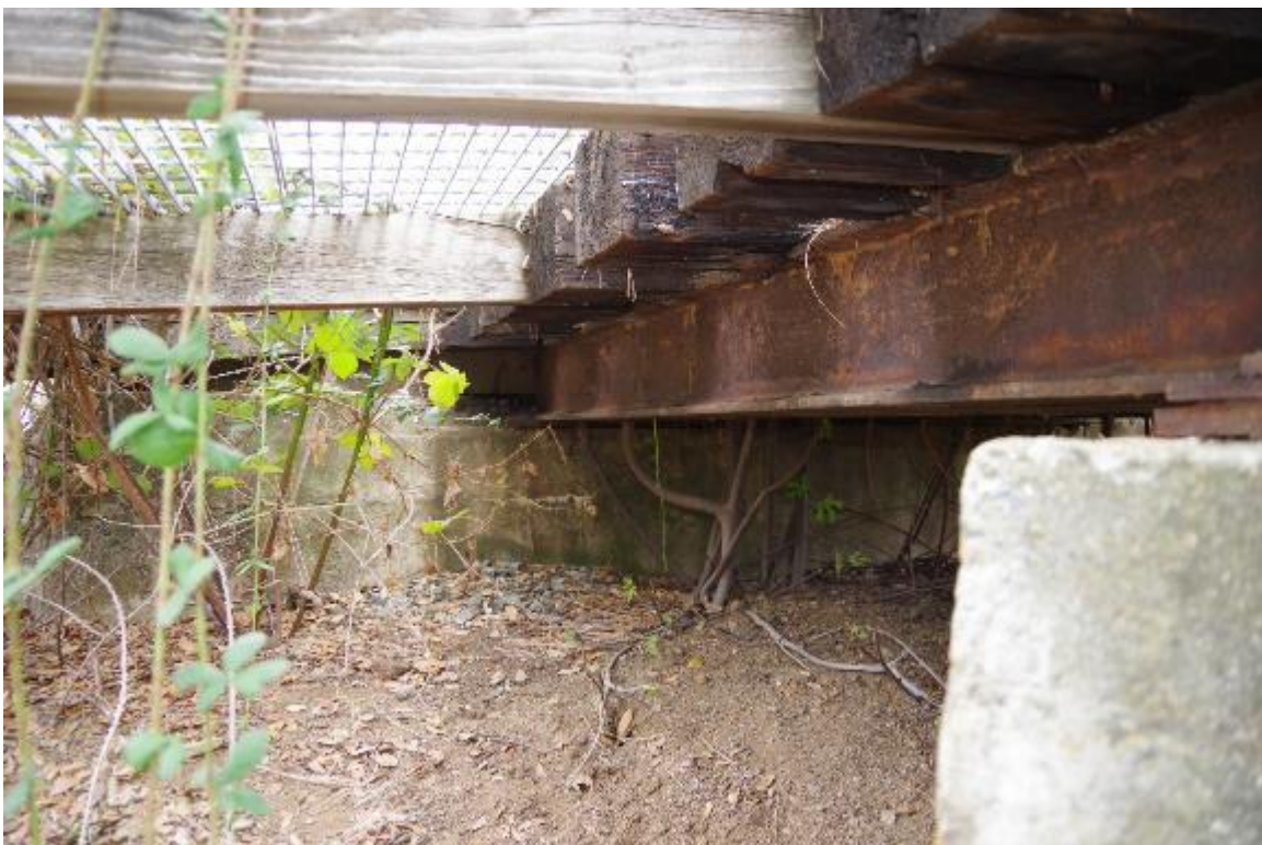
Photo 4: Vegetation growth underneath the bridge at abutment 1. Vegetation goes through the bridge as shown in Photo number 1.
