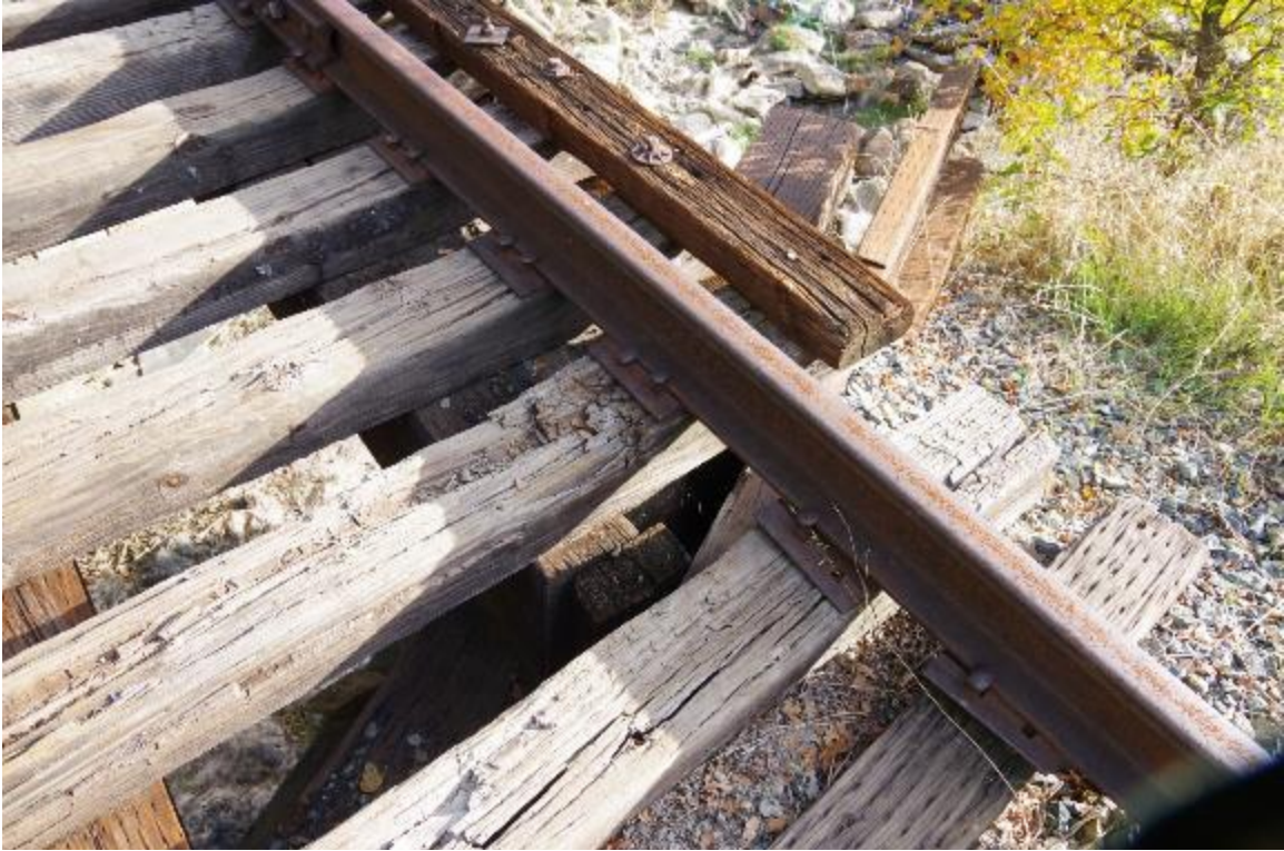
Photo 5: Closeup of railroad ties from abutment 1. Ties are in poor condition due to age and cracks observed. Tie keepers are also in poor condition.
