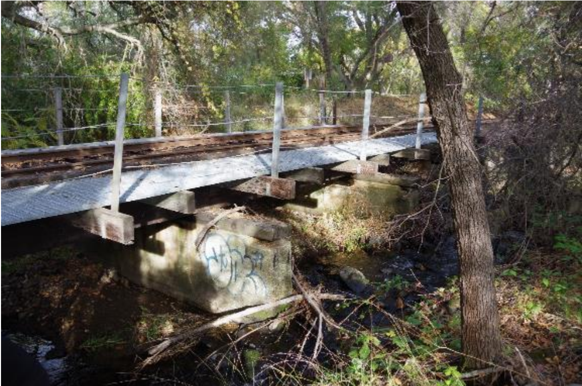
Photo 3: Bridge elevation view, shown is the right side of the track. Pier 2 and Pier 3 shown.
