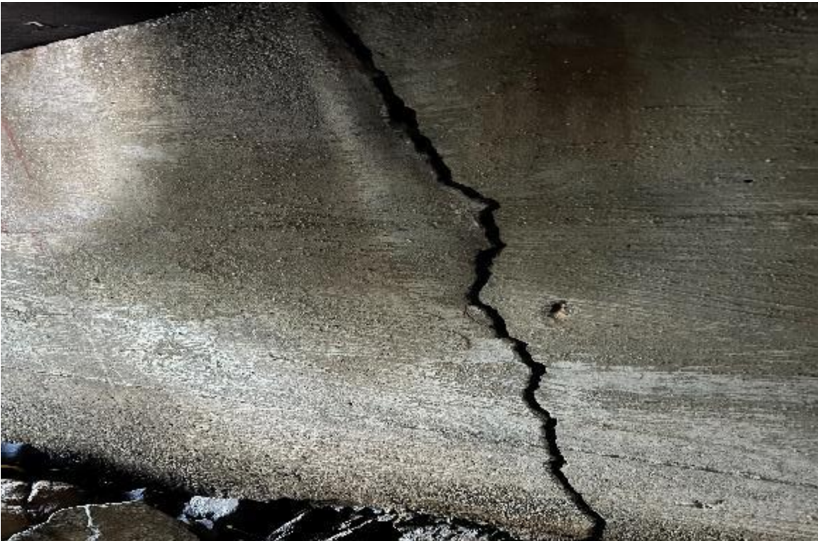
Photo 8: Second crack on Abutment 2
