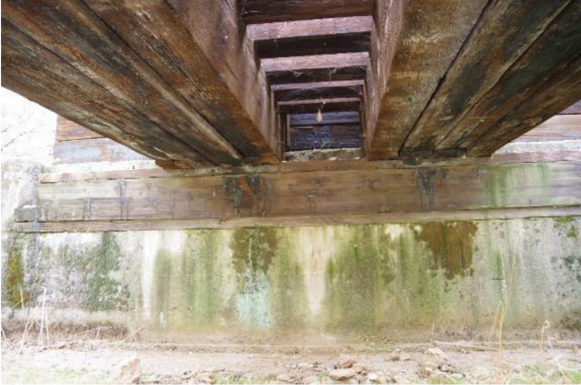
Photo 3: Typical abutment section view. Timber girders are in fair condition. Timber seat beams are also in fair condition. Exposed abutment height is 2.75 feet.
