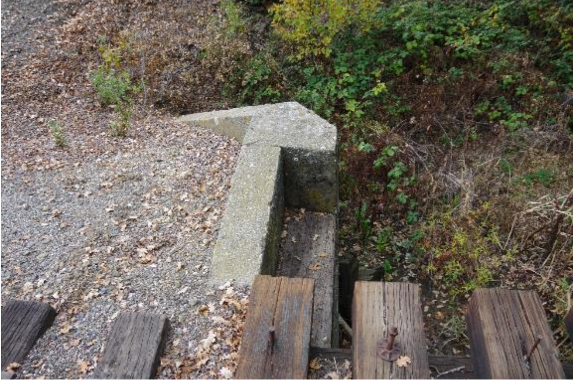
Photo 3: Top view of left side of abutment 1. Shown are the abutment seat and the corner of the abutment and wingwall.
