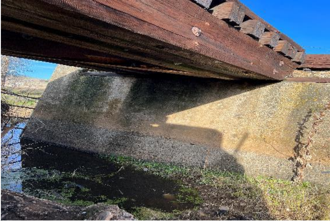
Photo 5: Bottom view of bridge girders. Fourth girder on the right side is broken, critical condition.
