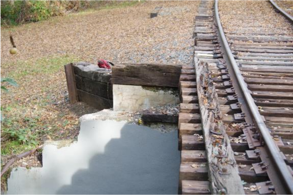
Photo 11: Closeup of left side of track. Tie keeper shown which is in critical condition. Also shown are Abutment 2 and small retaining wall.
