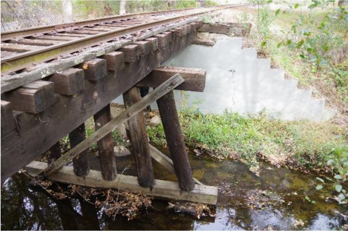
Photo 3: Pier 2 shown. Pier has 5 circular columns sitting on a timber beam. Beam sits on 4 concrete rectangular footings.
