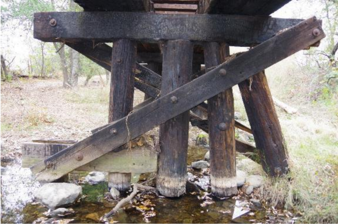
Photo 3: Closeup view of pier 2. One column is missing. Bent cap is charred and in poor condition. Column restrainers are in critical condition due to large crack.
