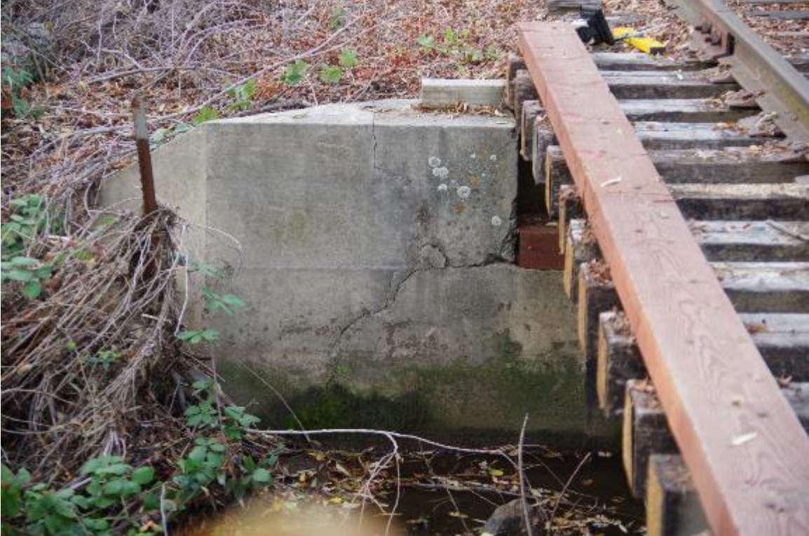
Photo 5: Abutment 1 closeup with a diagonal crack on left hand side.
