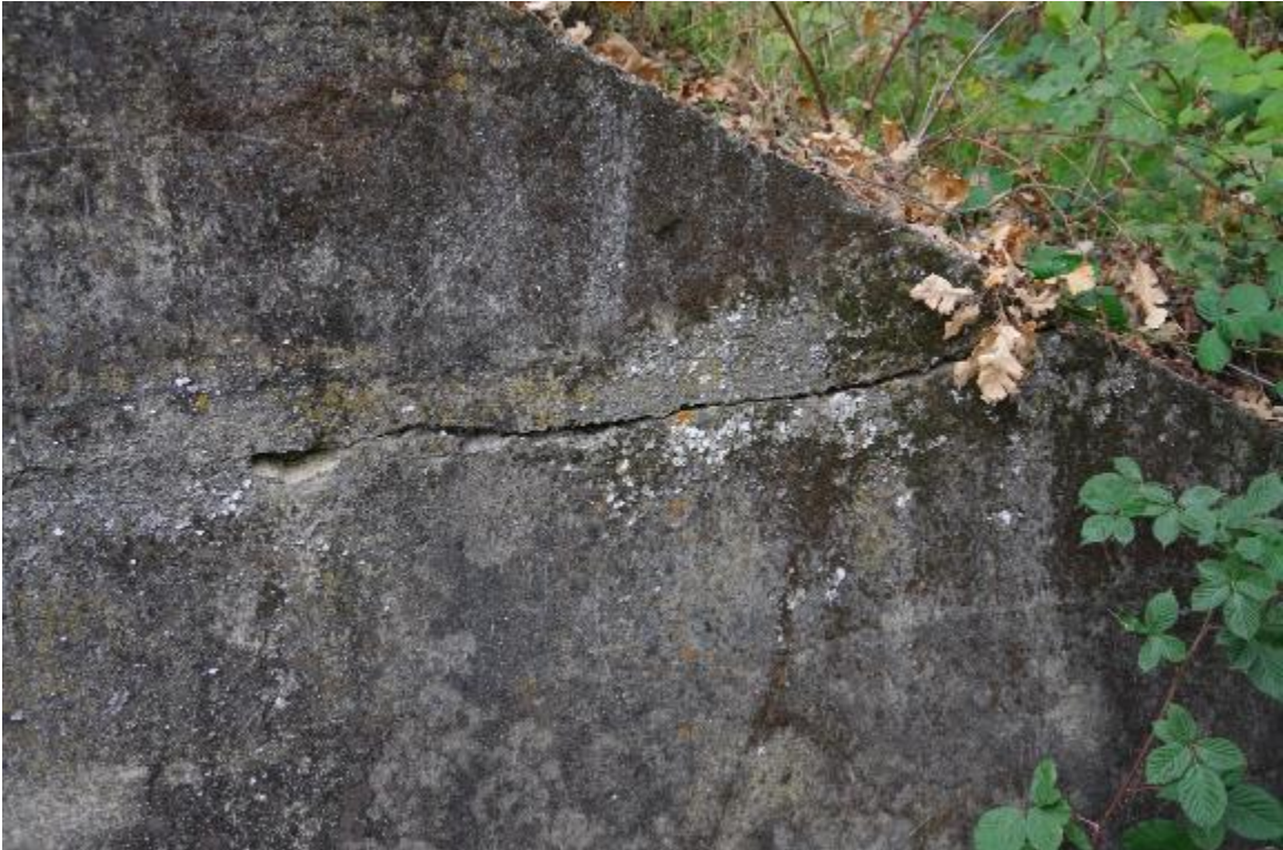
Photo 7: Abutment 2 right wingwall. Has a longitudinal 1/8" crack.
