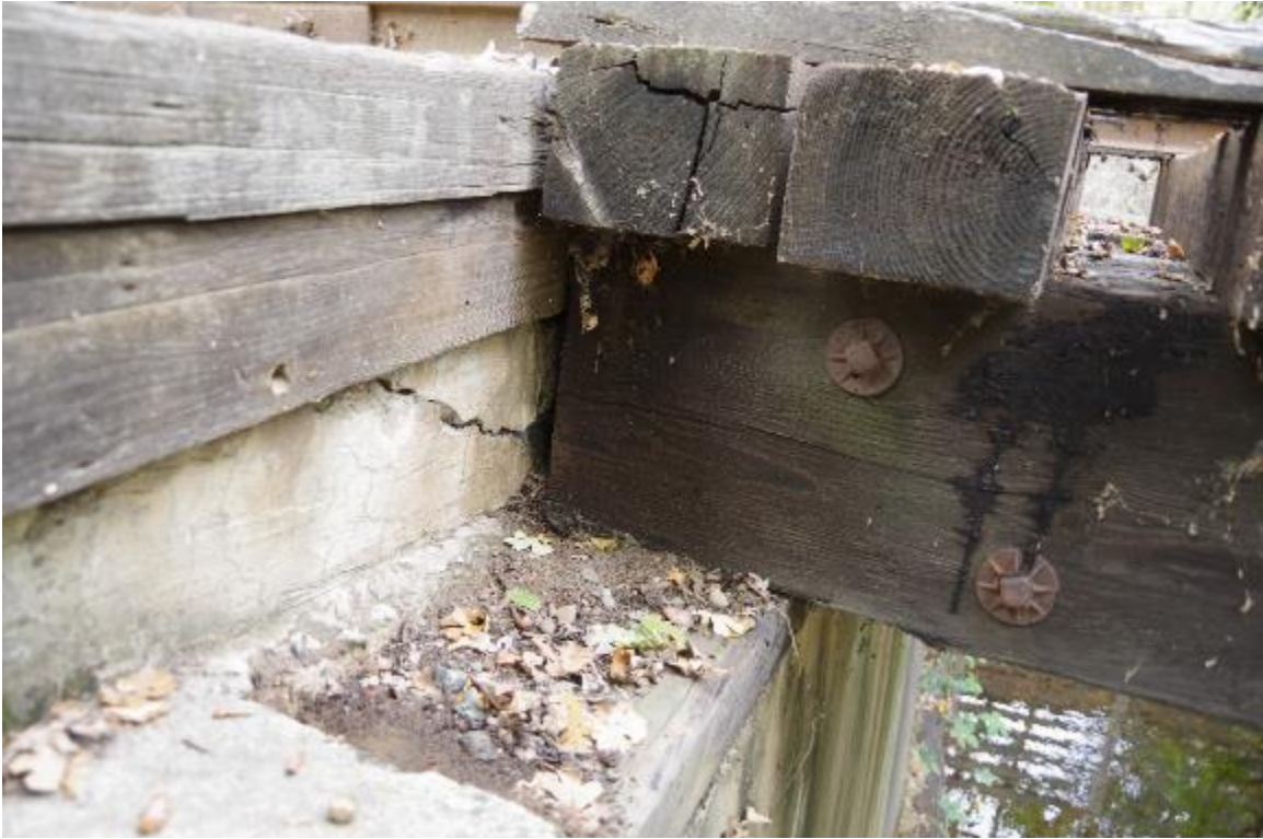
Photo 5: Timber beam to Abutment 1 connection. Beam sits on a 4"x12" sill beam. Crack shown at backwall at abutment 1.
