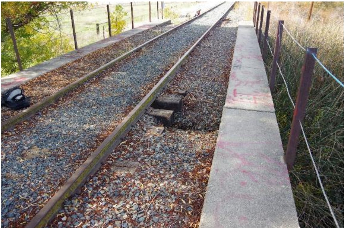
Photo 12: Loose ballast at an open joint
