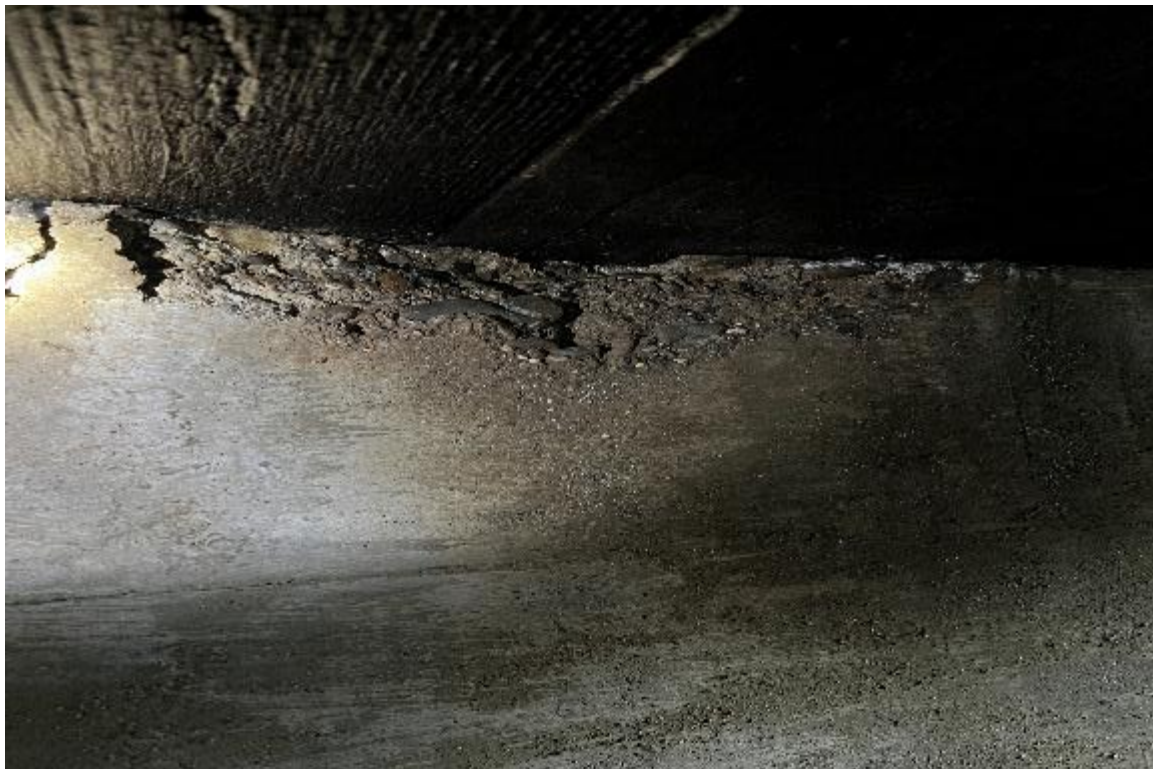
Photo 10: Concrete spalling at Abutment 1
