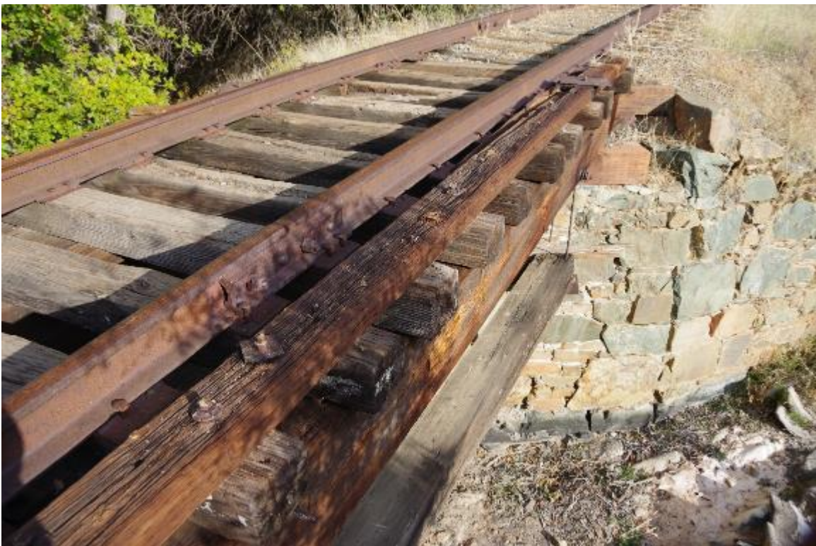
Photo 4: Close up view of track. Shown are the railroad ties, timber girders, tie keeper, and steel track.
