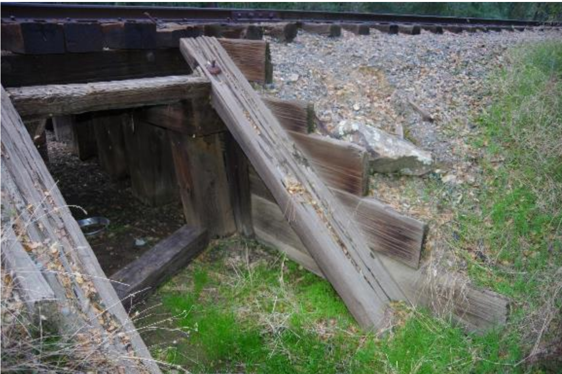
Photo 4: Closeup of the right side of Abutment 2. Timber lagging is in fair condition. Struts are in fair condition due to age.
