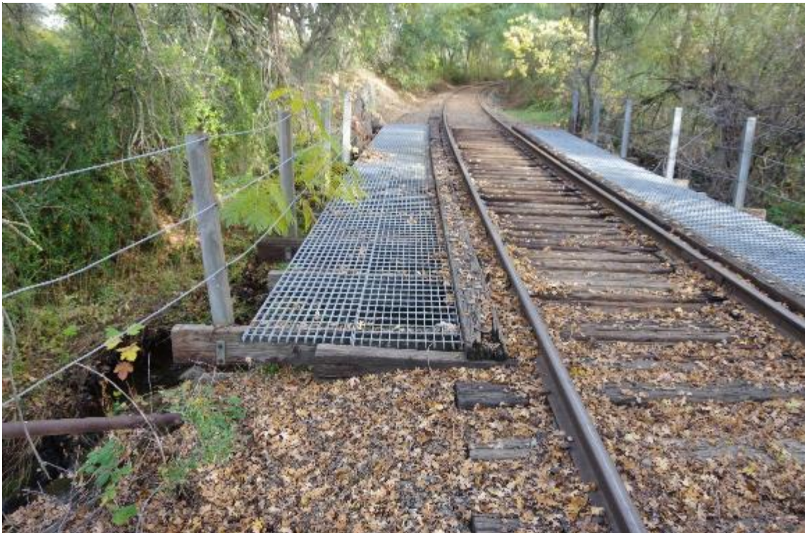
Photo 2: Closeup image of top view with walkway. Walkway supports, rails, tie keeper, and track shown.
