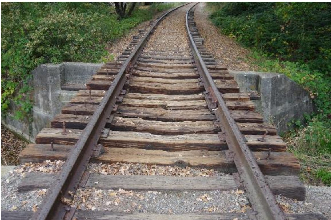
Photo 2: Close up view of top of bridge. Railroad ties are in poor condition. Span did not have tie keepers.
