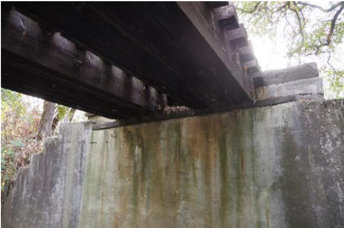
Photo 10: View of Abutment 1. No spalling observed at the abutment seat. A small crack can be seen underneath seat.
