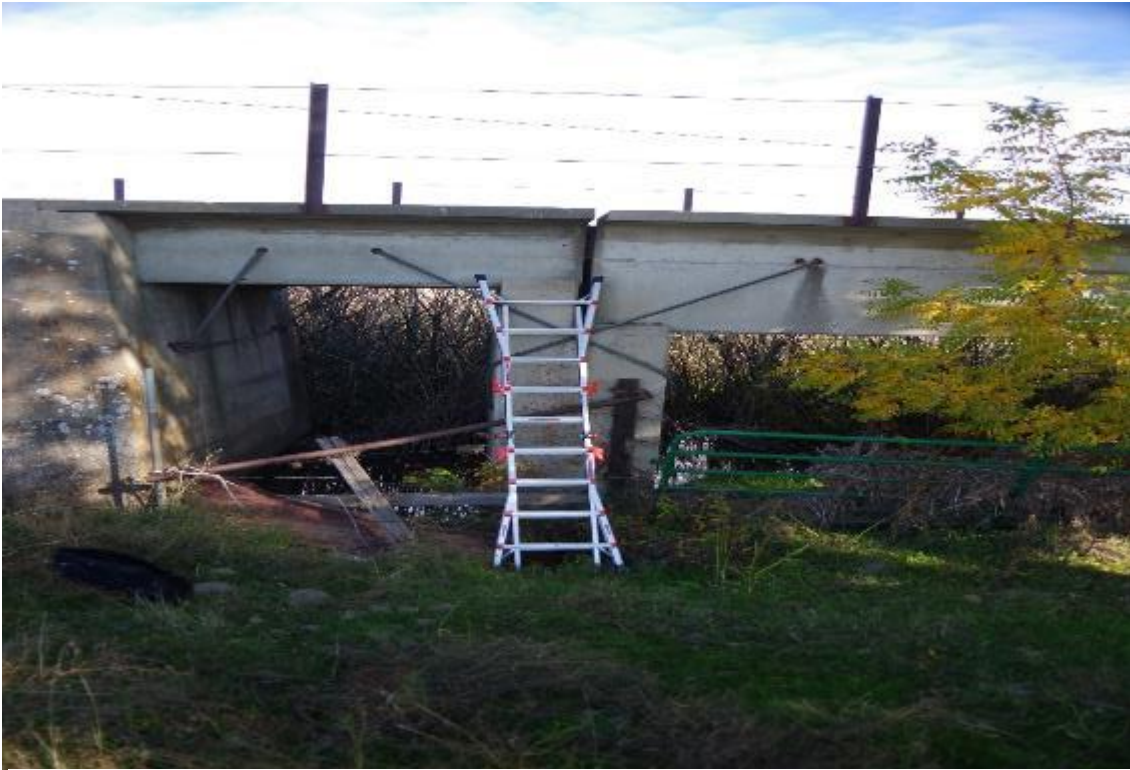
Photo 3: Elevation view of Abutment 1 and Pier 2, View from east side of the track. Abutment 1 is older than rest of the bridge.
