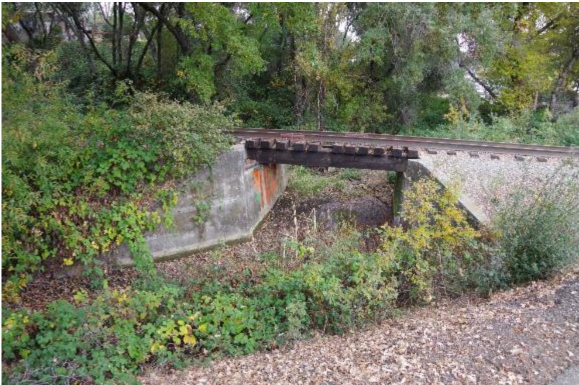
Photo 4: Bridge elevation view, left side of the track. Abutment 1(right) and Abutment 2 (left) shown. Span of bridge equals to 15 feet.
