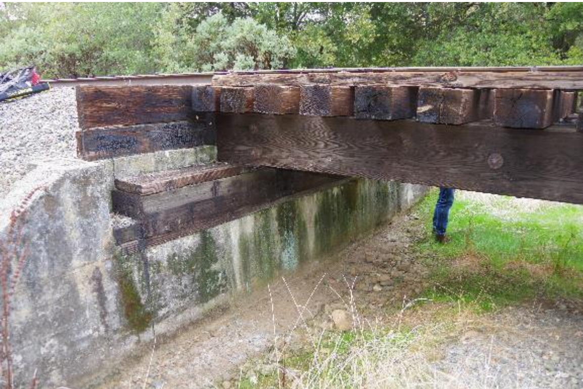
Photo 4: Girder to abutment 1 seat connection. Shown are the timber girders, railroad ties, sill beams, and headwalls.
