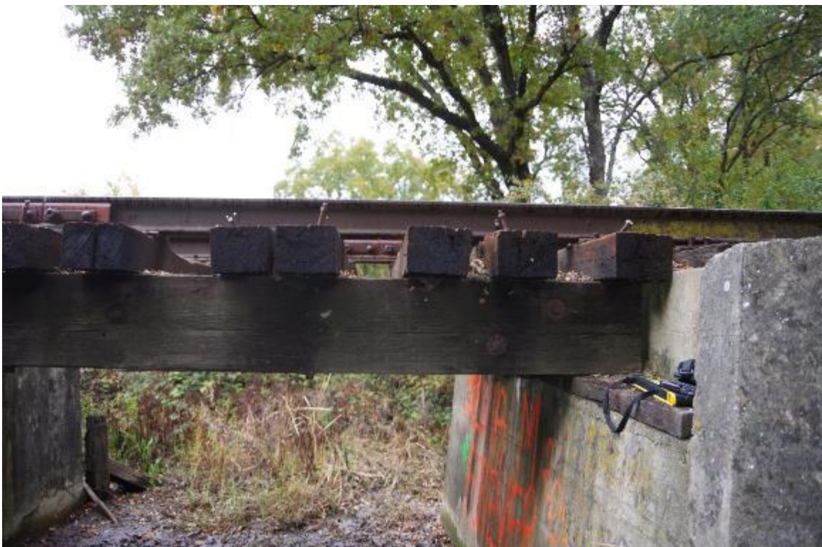
Photo 8: Right side elevation showing timber girders and rail road ties. Ties have unequal spacing. Ties and beams are in fair condition as no signs of cracking or decay were observed.
