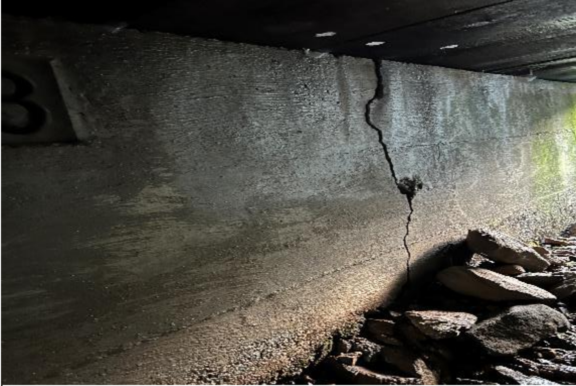
Photo 7: Diagonal crack on Abutment 2
