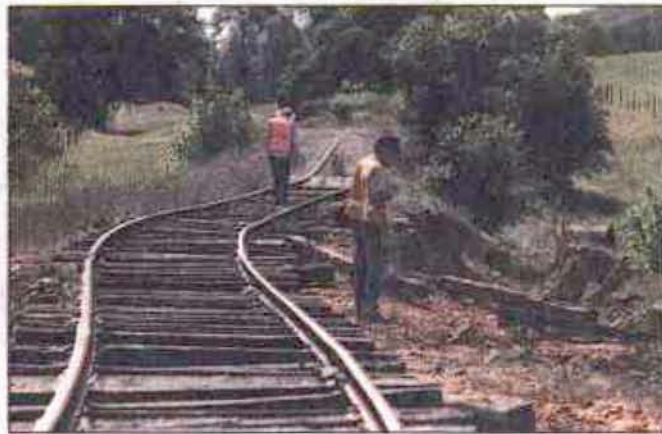
Rick Fuson, 72, left, and Al Onodera inspect sections of the Placerville Branch line by Latrobe Road damaged by floods. The line is largely usable, a group pushing tourist trips says.
