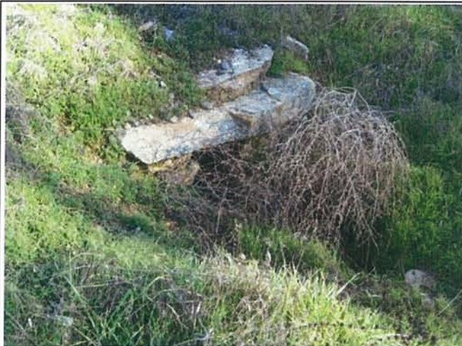
Feature 53: This feature is a small square stacked greenstone culvert. Facing SE. Frame 3422.
