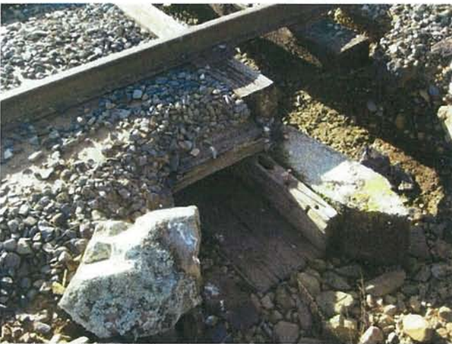
Feature 27: This feature is a wooden culvert and an absent culvert separated by a concrete diversion. Facing W. Frame 3347.
