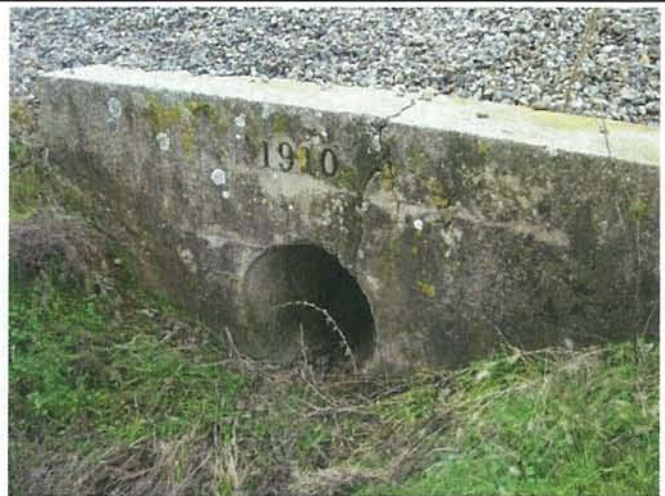
Feature 26: This feature is a poured concrete culvert with a date of "1910" stamped onto the face of the concrete. Facing S. Frame 3338.
