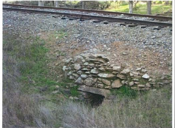
Feature 58: This feature is a greenstone culvert with multiple courses of greenstone stacked on top. Facing N. Frame 3433.
