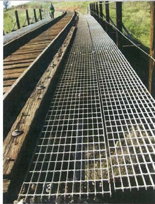
Feature 89: Bridge #08 Deer Creek Bridge. This feature is an historic era bridge built in 1913. It is constructed of two simple span steel plate girders with an open timber deck and steel open grate walkways on reinforced concrete abutments. Track ties of 10 inches x 12 inches x 10 feet rest directly atop the steel stringers and support in turn tie plates and the two running rails. The track is of conventional bolted rail construction. Stone masonry wing walls protect the upstream and downstream ends of both abutments. It is 72.5 feet long and 16 feet wide. Photo facing W. Frame 3400.
