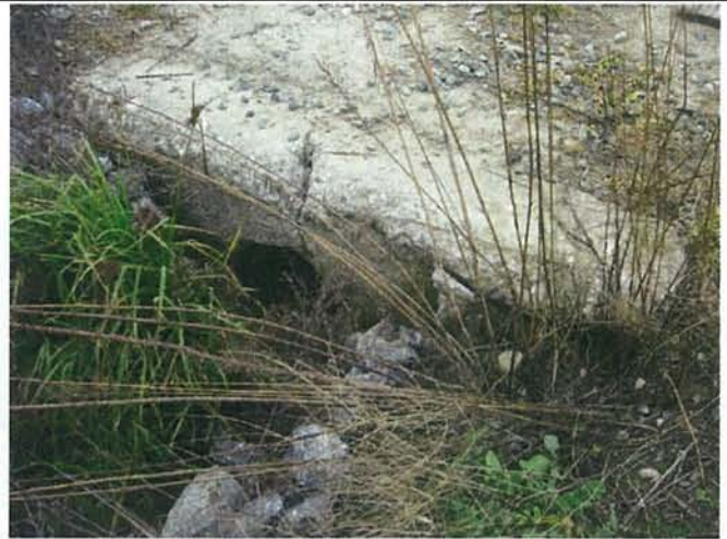
Feature 22: This feature is a metal culvert inside a poured concrete case. Facing N. Frame 3329.
