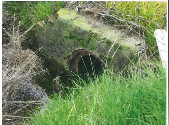
Feature 24: This feature is a culvert of brick encased in mortar surrounding a brown glazed ceramic culvert with "...LINCOLN, CA" stamped on the mouth of the ceramic. Facing S. Frame 3332.
