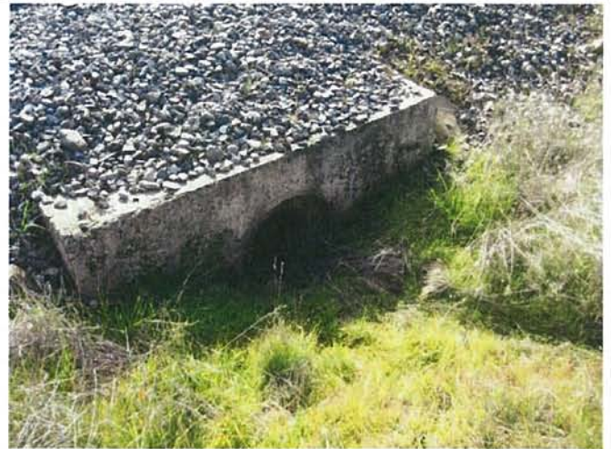
Feature 70: This feature is a concrete culvert with a round opening. Facing S. Frame 3469.
