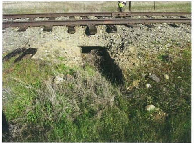
Feature 86: This feature is a burnt out wooden culvert. Facing ENE. Frame 3494.
