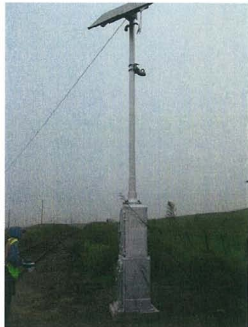
Feature 20: This feature is an electric box with a modern solar panel attached. Facing NW. Frame 3327.
