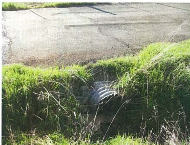
Feature 4: This feature is a corrugated metal culvert. Road repaved above. Facing W. Frame 3348.
