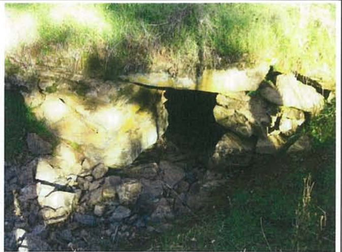
Feature 46: This feature is a large stacked greenstone culvert. Facing NE. Frame 3415.
