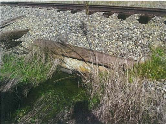
Feature 75: This feature is a greenstone culvert with railroad ties. Facing N. Frame 3475.
