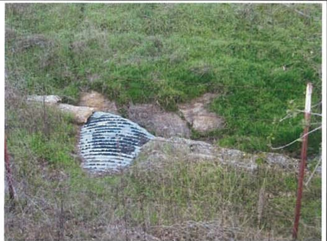
Feature 62: This feature is a very large corrugated metal culvert with cement sandbag support. Facing NE. Frame 3441.
