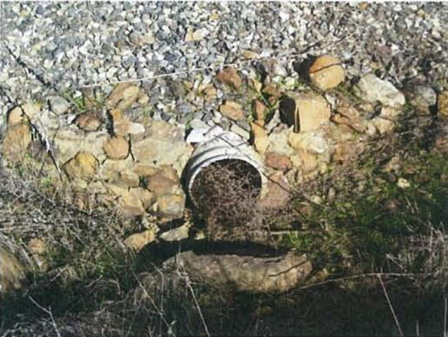
Feature 87: This feature is fieldstone and loose mortar around a corrugated metal culvert. Facing ENE. Frame 3495.
