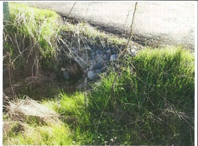
Feature 6: This feature is a corrugated metal steel culvert. Facing W. Frame 3352.
