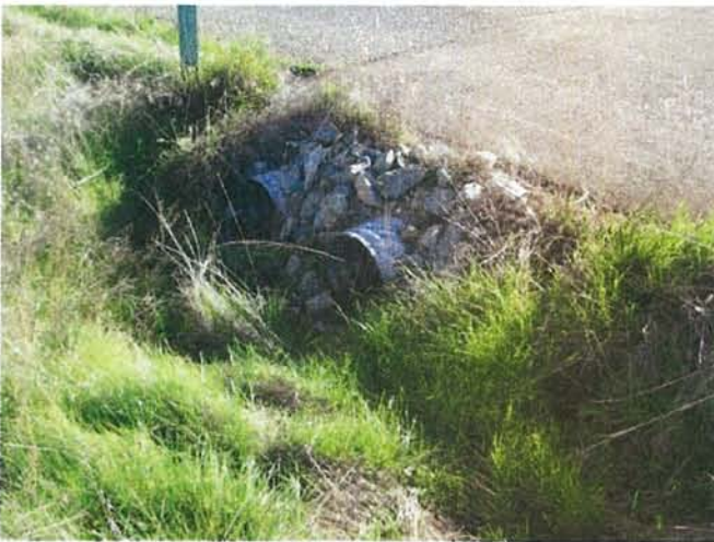
Feature 7: This feature is two galvanized metal culverts. Road repaved above. Facing S. Frame 3354.
