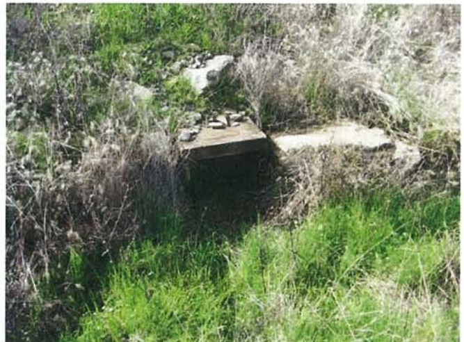
Feature 72: This feature is a small square wooden culvert. Facing WSW. Frame 3471.
