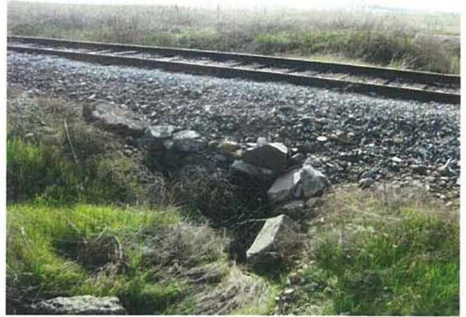
Feature 6: This feature is rock and steel pipe culvert. Facing W. Frame 3305.
