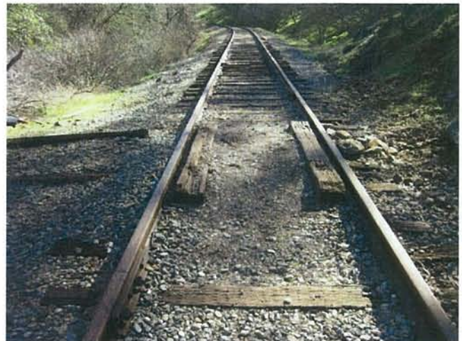
Feature 38: This feature is a wooden de-railer track at which hand cars come off the track. It is comprised of one set of parallel embedded railroad ties in between the tracks themselves that are nine feet long, and two parallel embedded railroad ties 5 feet apart coming jutting out from the track for 14 feet. Facing ESE. Frame 3396.
