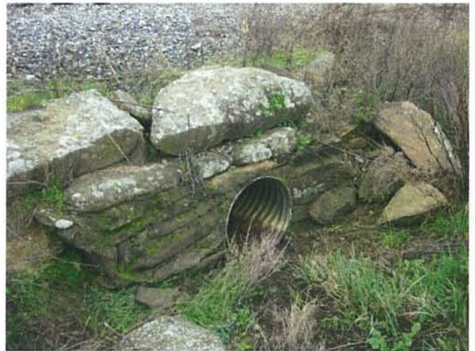
Feature 14: This feature is a copper steel corrugated metal culvert surrounded by rocks with mortar between the rocks and over the pipe itself. Facing SW. Frame 3319.
