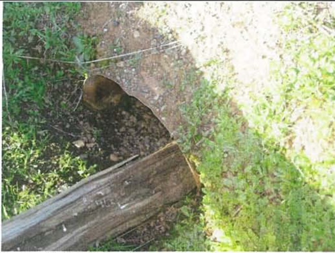
Feature 9: This feature is corrugated galvanized steel culvert. Repaved above. Facing NW. Frame 3361.
