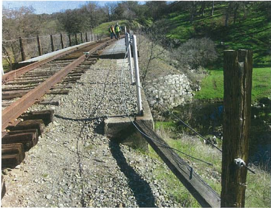
Figure 16. Deer Creek Bridge looking east at north end of Ben Bolt Ridge.
