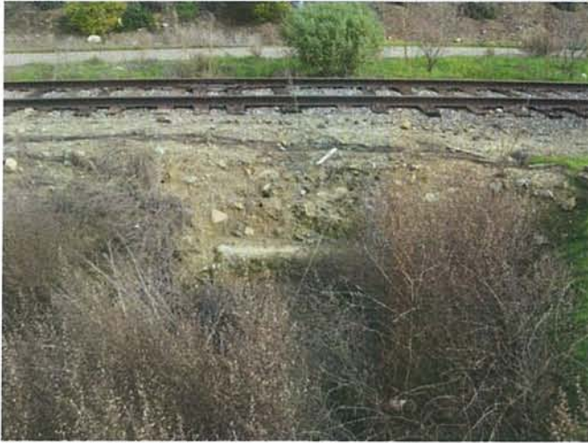
Feature 1: This feature is a concrete capped corrugated metal culvert. Facing E. Frame 3297.
