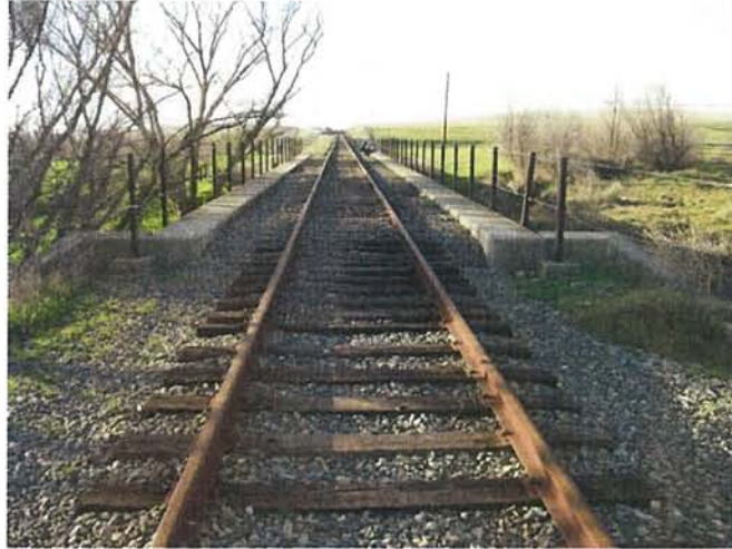
Feature 91: This feature is a concrete bridge 134 feet long and 17 feet wide with a 2.5 foot wide concrete foot path on either side, and a railing made of 3.5 foot tall metal posts strung through with thick wire. It has 4 concrete piers and is supported by concrete abutments. Photo facing NW. Frame 3364.
