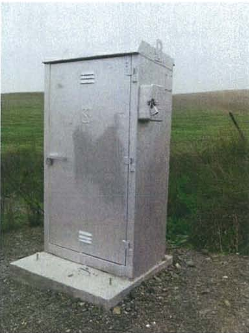
Feature 19: This feature is a box containing electrical signal reader. Facing N. Frame 3326.
