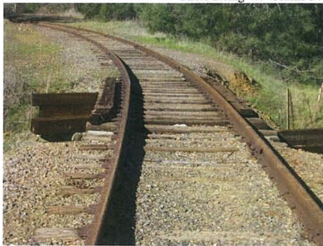
Feature 90: Bridge #9 Deer Creek Bridge. This feature is an open deck timber stringer span without walkways on a stone masonry struted abutments. Trackties of 7 inches x 9 inches x 8 feet rest directly atop the stringers and support in turn tie plates and the two running rails and 3x8 timber gaurds. Timber 12x12 struts and ledgers brace each abutment breast wall. It is 20.8 feet long and 7.5 feet wide. Photo facing NW, frame 3382.
