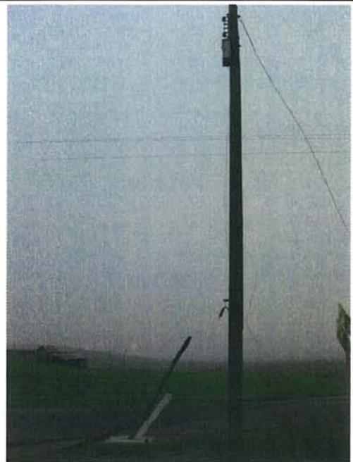
Feature 18: This feature is a concrete foundation and distribution pole for an electrical signal. Facing SW. Frame 3325
