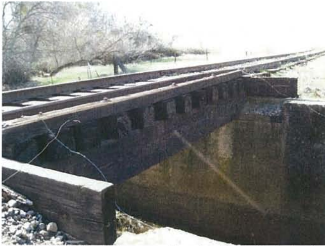
Feature 88: Bridge #07 unnamed creek bridge. This feature is an open deck timber stringer span bridge without walkways on reinforced poured concrete abutments, built in 1904. Track ties of 7 inches x 9 inches x 8 feet rest directly atop the stringers and support in turn tie plates and the two running rails. The track is of conventional bolted rail construction. It is 8 feet wide and 15.5 feet long. Photo facing SSW. Frame 3463.
