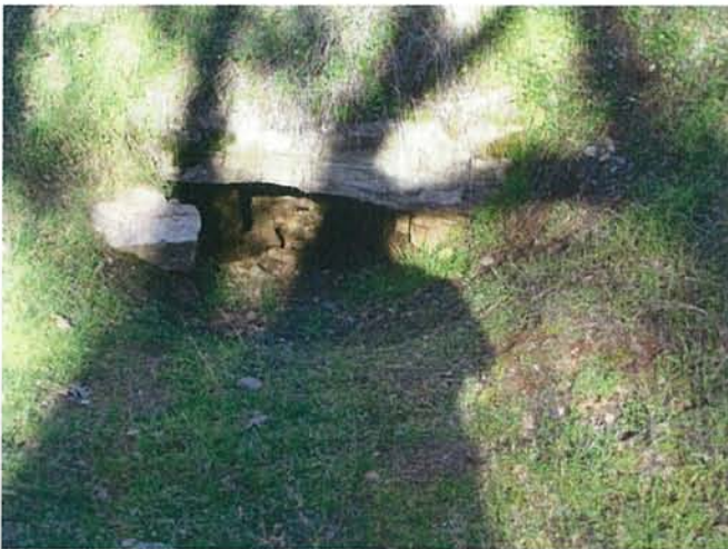
Feature 47: This feature is a large, stacked greenstone culvert. Facing NE. Frame 3416.
