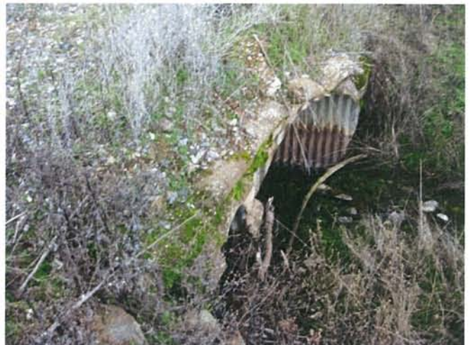
Feature 64: This feature is a double corrugated metal culvert with concrete sandbags. Facing N. Frame 3444.
