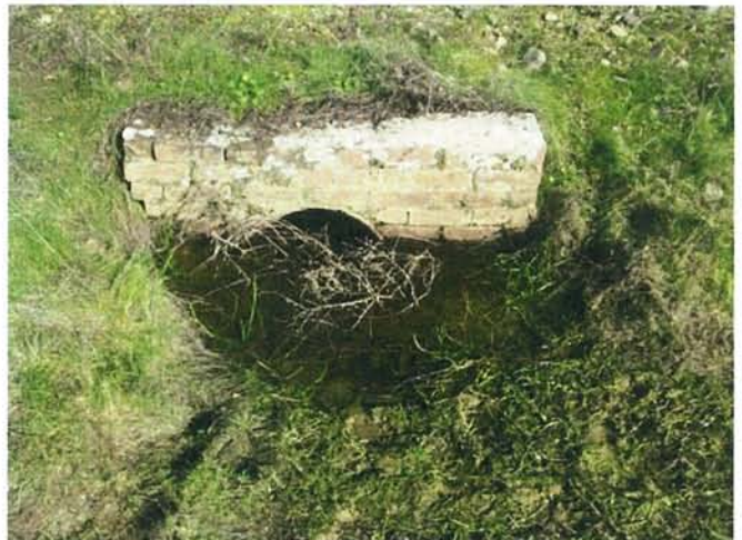
Feature 84: This feature is a clay culvert surrounded by brick and mortar. Facing ENE. Frame 3491.
