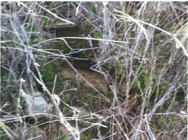
Feature 67: This feature is a tiny collapsed culvert. Facing SSE. Frame 3454.
