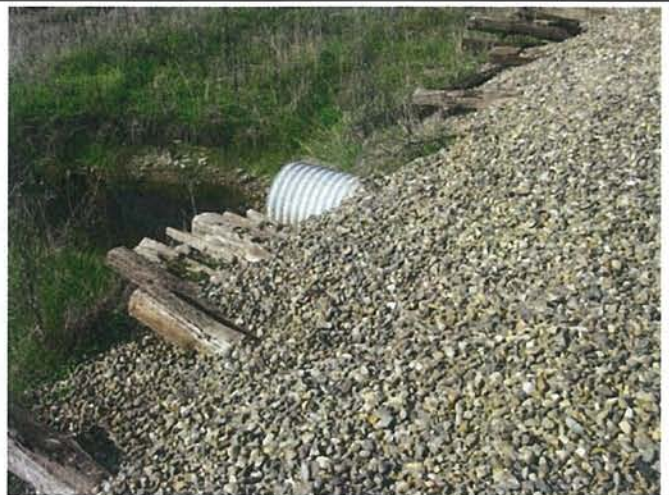
Feature 74: This feature is a corrugated metal culvert with railroad ties above for erosion control. Facing W. Frame 3474.
