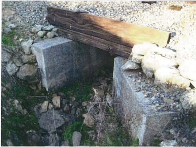
Feature 61: This feature is a concrete and wooden culvert. Facing N. Frame 3438.
