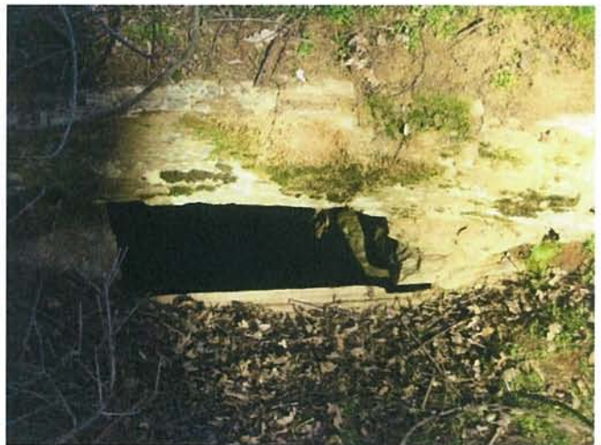
Feature 48: This feature is a rectangular stacked greenstone culvert. Facing NE. Frame 3417.
