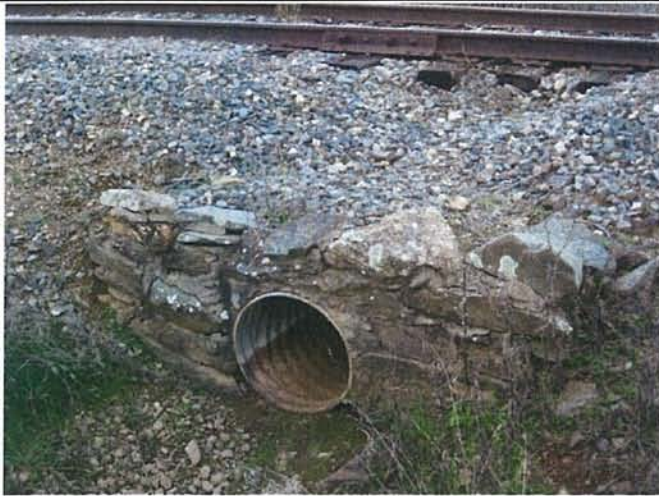
Feature 65: This feature is a corrugated metal culvert encased in mortared courses of angular rocks. Facing NE. Frame 3445.
