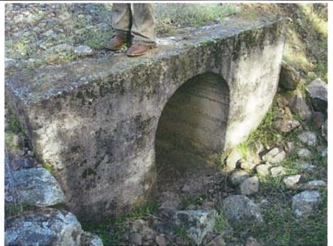
Feature 34: This feature is a poured concrete arched culvert. Facing N. Frame 3389.
