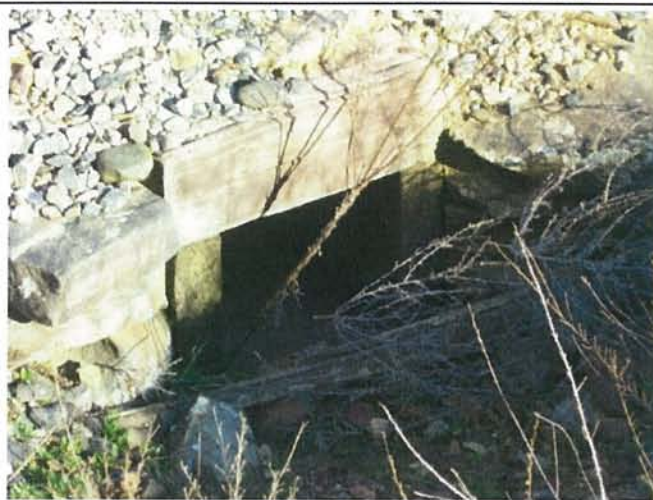
Feature 54: This feature is a very small wooden culvert. Facing E. Frame 3423.
