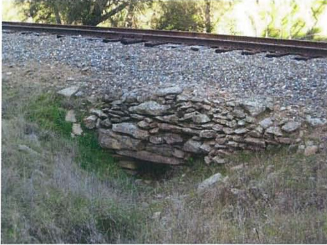
Feature 57: This feature is a stacked greenstone culvert with multiple courses of greenstone stacked on top. Facing N. Frame 3432.
