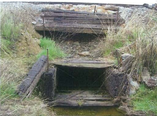
Feature 11: This feature is a wooden culvert constructed of railroad ties with erosion control of railroad ties above. Facing South. Frame 3314.
