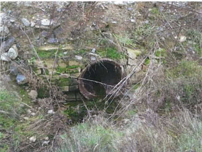
Feature 15: This feature is a brown glazed ceramic culvert surrounded by brick. Facing WSW. Frame 3320.
