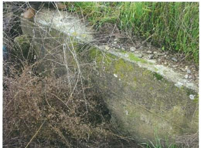
Feature 16: This feature is a poured concrete culvert with a date of "1910" stamped into the face of the concrete. Facing S. Frame 3321.
