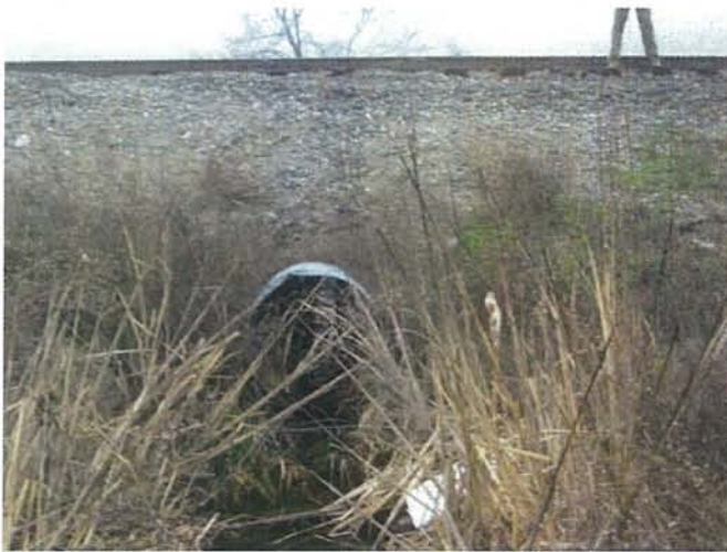
Feature 9: This feature is a corrugated steel culvert surrounded by rock. Facing north
