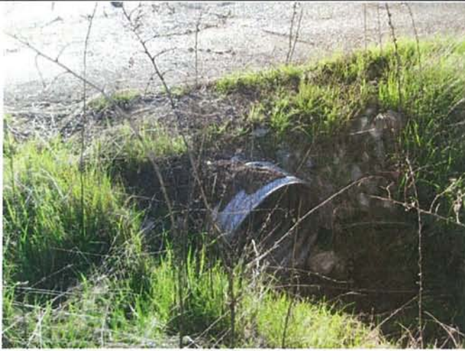
Feature 5: This feature is a corrugated metal culvert. Road repaved above. Facing W. Frame 3350.
