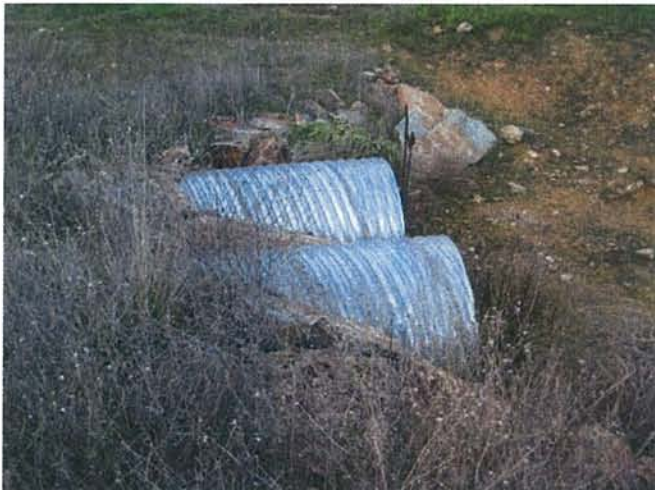
Feature 63: This feature is a double corrugated metal culvert. Facing NE. Frame 3443.
