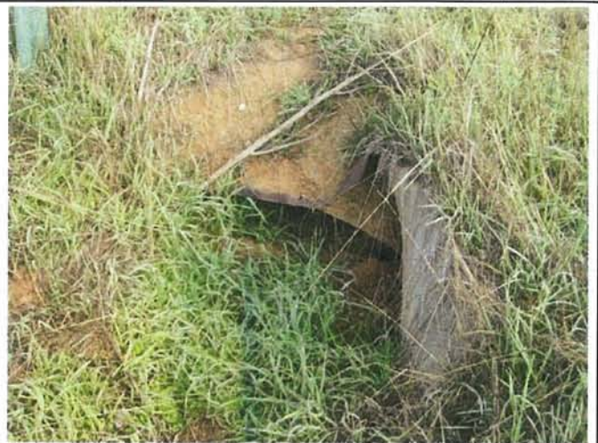
Feature 10: This feature is a corrugated sheet metal culvert. Facing N. Frame 3378.
